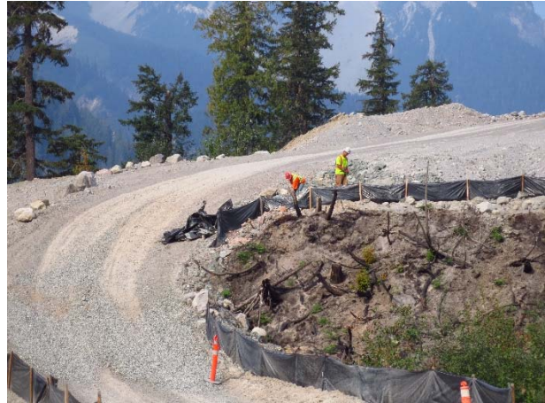
Photo 2 – Replacement of silt fencing protection at the ASTR03 road culvert crossing. (August 27, 2015).
