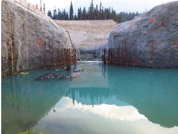
Photo 3 – Flooded conditions within the ULRHEF upstream tunnel and intake structure prior to dewatering (August 27, 2015).
