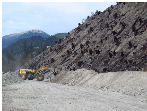
Photo 14 – Construction of a berm to protect the ULRHEF powerhouse access road from landslide and falling material risks (August 26, 2015).
