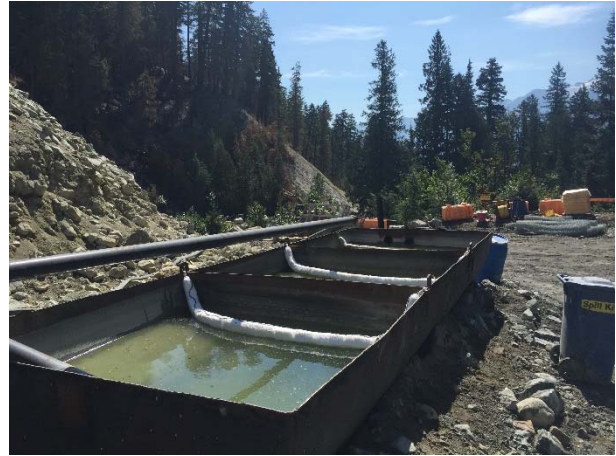
Photo 8 – Replacement of the oil absorbent booms in the oil/water separator (August 12, 2015).
