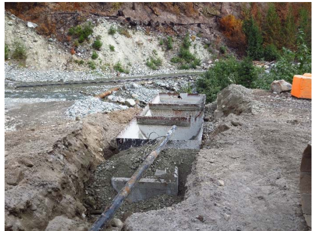
Photo 10 – The oil/water separator was moved to create more space at the downstream tunnel portal entrance (August 28, 2015).
