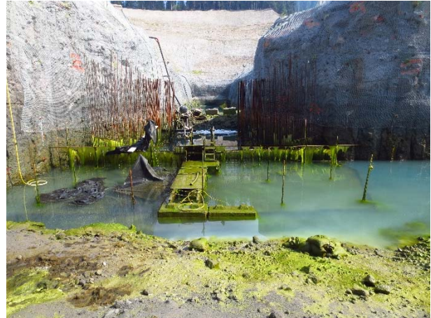
Photo 4 – Conditions of the form work and rebar for the intake structure following dewatering (August 27, 2015).
