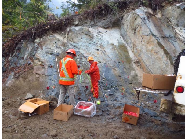
Photo 18 – Blast preparations at the Ryan River bridge approach. A hydrophone and seismograph was installed to monitor in-stream acoustic pressure during the blast (August 28, 2015).
