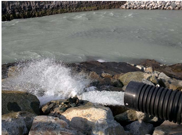
Photo 5 – Clean water discharging to the Lillooet River from the flooded tunnel and intake work area following confirmation that water met BCWQGs (August 27, 2015).
