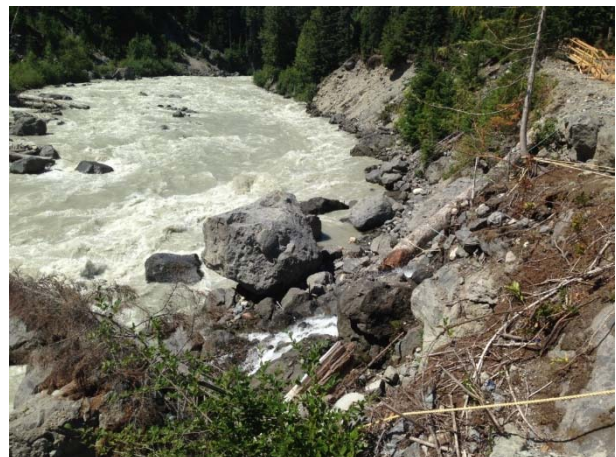
Photo 8 – ULRHEF powerhouse sump dewatering to Lillooet River (July 1, 2015).
