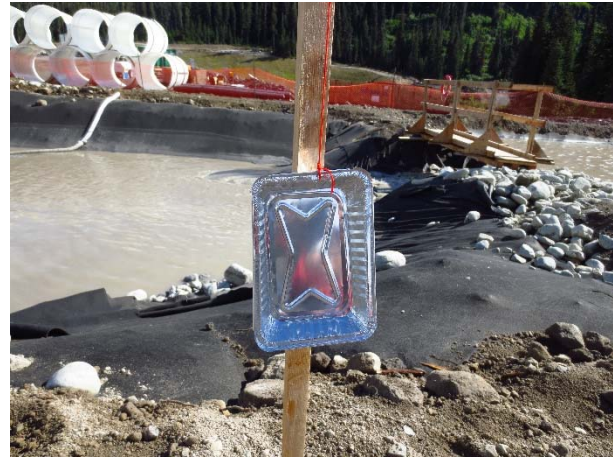
Photo 8 – Bird deterrent measures installed at ULRHEF intake and upstream tunnel portal sediment basins (June 20, 2015).
