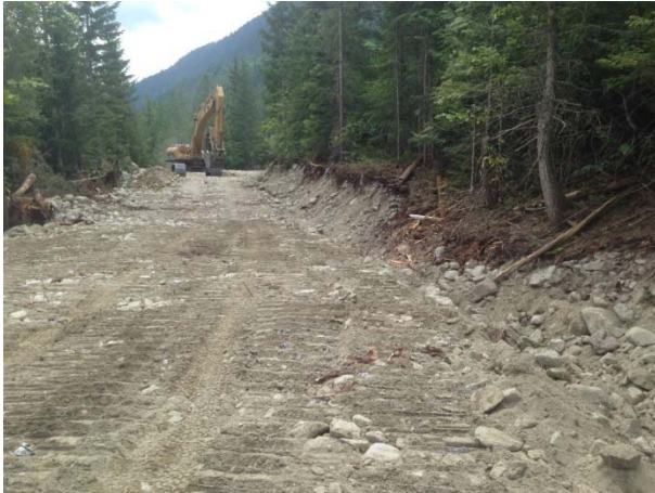
Photo 20 – Ditching and road works on Ryan South Main near stream 261a (June 18, 2015).
