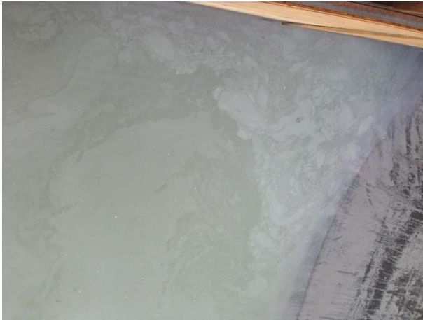
Photo 7 – Oil residue visible in ULRHEF intake and upstream tunnel portal sediment basins (June 19, 2015).
