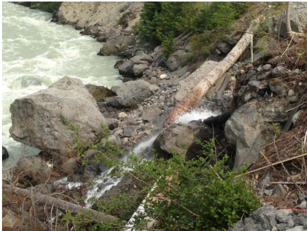
Photo 15 – ULRHEF powerhouse sump discharging to the Lillooet River (June 18, 2015).
