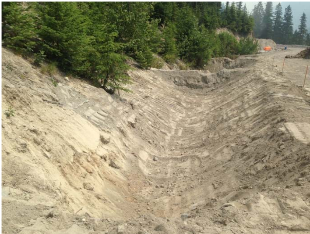
Photo 11 – New downstream tunnel portal settling pond site on penstock alignment at 2+800 (June 17, 2015).
