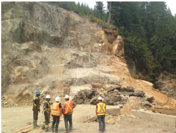
Photo 16 – Conditions at BDRHEF intake following blast above crane pad (June 16, 2015).
