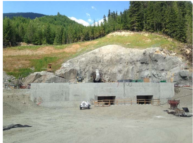
Photo 23 – Backfilled area adjacent to the BDRHEF powerhouse to be used as a crane pad (May 26, 2015).
