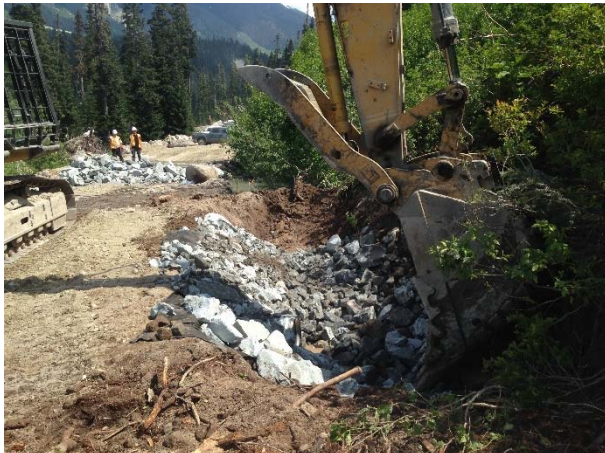
Photo 3 – Ditch and culvert inlet armoring during culvert installation at KM 49.7 of the ULRHEF intake access road (May 26, 2015).
