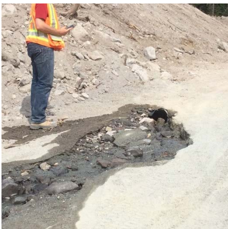
Photo 10 – Broken pipe outletting from the ULRHEF intake sediment ponds was repaired on May 30, 2015 (May 28, 2015).
