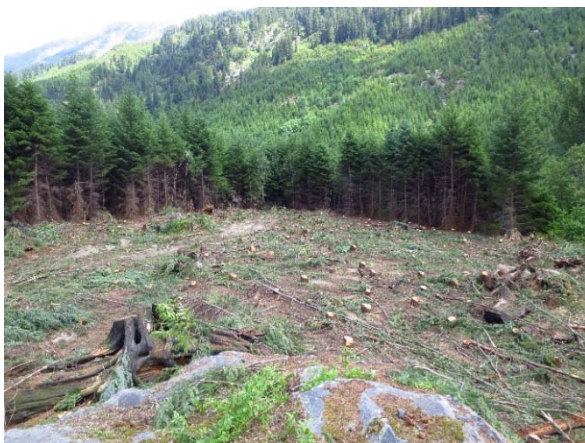
Photo 5 – Clearing completed at the future permanent PAG storage area near KM 42 of the Lillooet River FSR (May 30, 2015).
