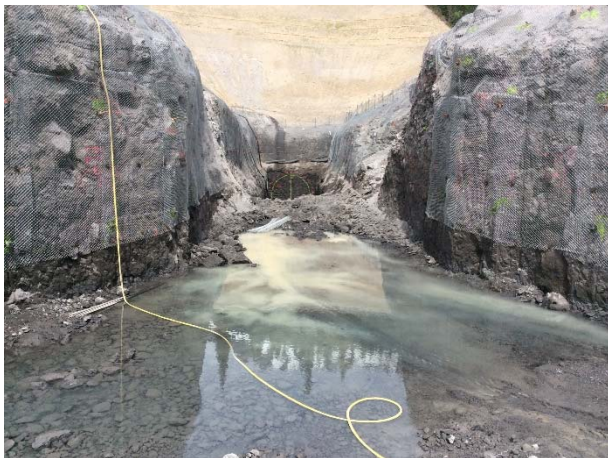
Photo 8 – Work on hold at the upstream tunnel portal and intake area. Clear seepage within the intake excavation was directed to the Lillooet River (May 28, 2015).
