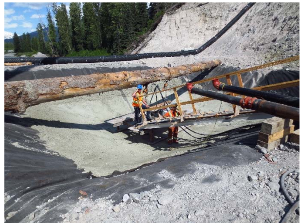
Photo 9 – Repairs completed on the lower sump, which included re-lining with impermeable membrane and a concrete skim coat (May 30, 2015).
