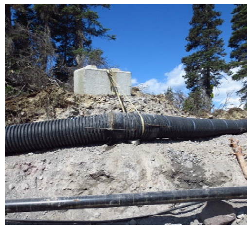
Photo 11 – Repairs completed on the outlet pipe that directs water that meets BCWQGs to the Lillooet River (May 30, 2015).
