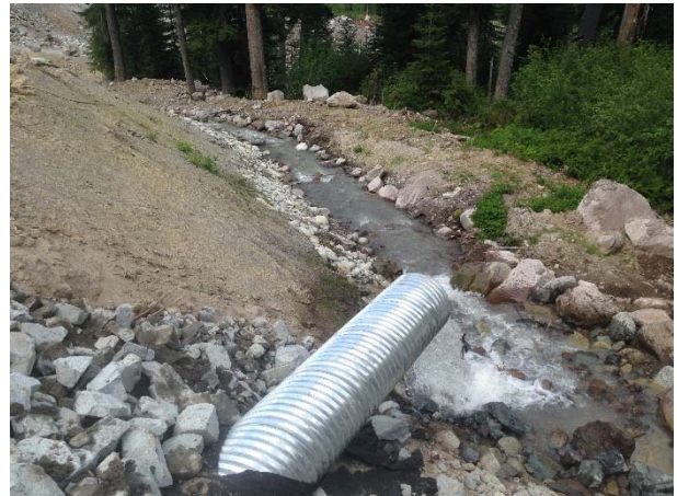
Photo 4 – Culvert outlet during commissioning of the newly installed culvert at KM 49.7 of the ULRHEF intake access road (May 26, 2015).
