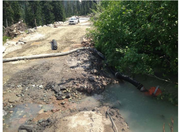
Photo 2 – Diversion pump and overflow ditch installed to ensure culvert installation works were performed in the dry at KM 49.7 km the ULRHEF intake access road (May 26, 2015).
