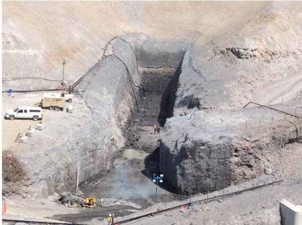
Photo 6 – Current conditions at the ULRHEF intake and tunnel portal work areas (May 27, 2015).
