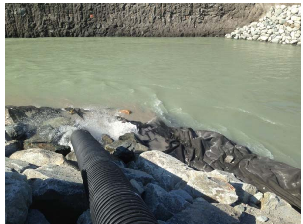
Photo 8 – Sediment-laden water discharged to Lillooet River (May 17, 2015).
