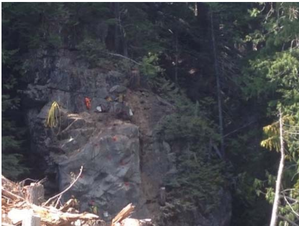
Photo 22 – Rope access crews conduct scaling works on the right bank at the BDRHEF intake (May 18, 2015).
