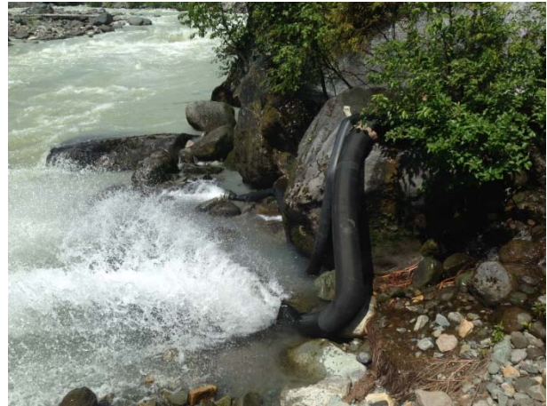
Photo 21 – ULRHEF powerhouse sump dewatering to Lillooet River (May 19, 2015).
