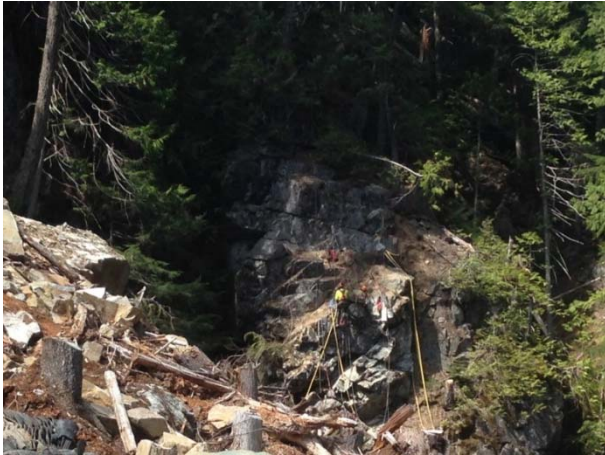
Photo 20 – Rope access crews conduct scaling works on right bank at BDRHEF intake (May 11, 2015).
