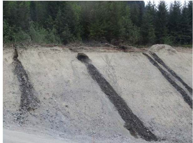
Photo 14 – Runoff flowing down penstock excavation slope at 4+050 (May 13, 2015).
