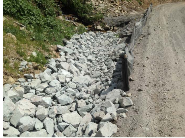
Photo 2 – Ditch maintenance and silt fencing repair at a tributary crossing near 43.5km on the Lillooet River FSR (May 12, 2015).
