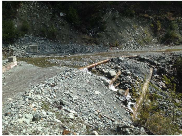
Photo 8 – Conditions at Truckwash Creek (May 1, 2015)
