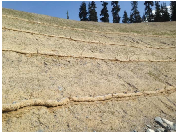
Photo 5 – Intake left bank slope with curlex logs and hydroseeding to prevent rilling and erosion; hydroseeded grass sprouting on top of bank (May 2, 2015).
