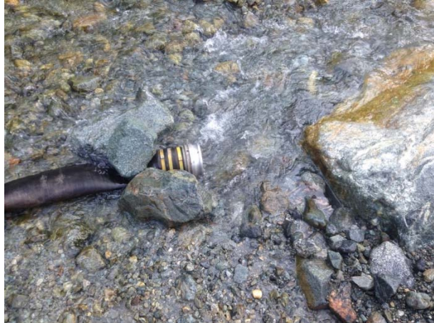
Photo 10 – Hose positioned in Truckwash Creek for dewatering of ULRHEF downstream tunnel portal (May 1, 2015).
