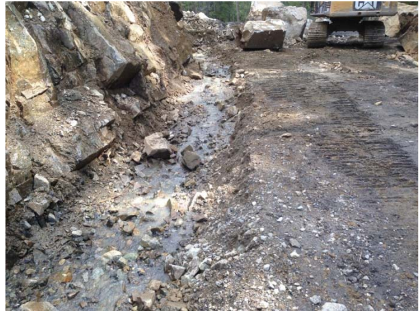
Photo 17 – Ditch water with clear flows at 3.75km on BDRHEF intake access road (May 2, 2015).
