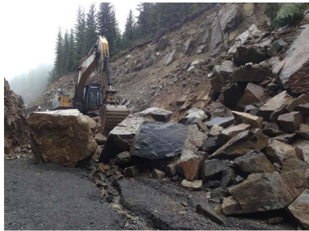
Photo 15 – Road clearing and bank stabilization works at 4.75km on BDRHEF intake access road (May 1, 2015).
