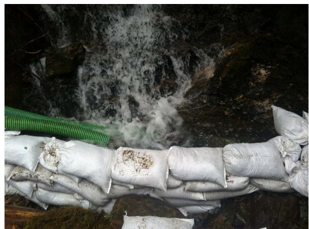
Photo 13 – Sandbag dam and pumps used for worksite isolation at MB50 in Segment 12 (April 22, 2015).
