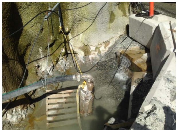
Photo 4 – BDRHEF tunnel discharge catchment and pump inlet (April 8, 2015).
