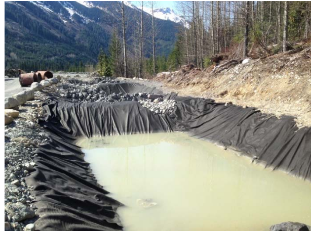
Photo 6 – BDRHEF powerhouse settling ponds; water infiltrating to ground in first cell (April 8, 2015).
