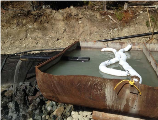
Photo 5 – Oil water separator discharging to settling ponds (April 8, 2015).
