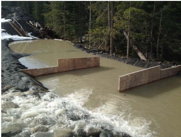
Photo 5 – ULRHEF powerhouse settling ponds during French drain excavation for backfill works (April 1, 2015).
