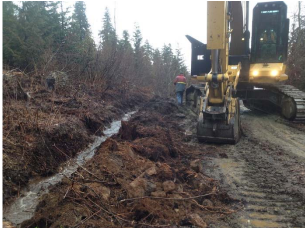
Photo 13 – Excess water not handled by the pumps at MB27 was diverted down ditch where it discharged to vegetation (March 30, 2015).
