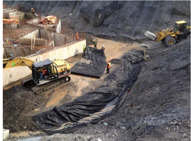
Photo 4 – Backfill works at ULRHEF powerhouse with geotextile fabric placed for French drain (April 1, 2015).
