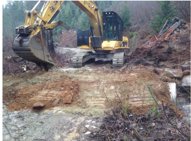
Photo 14 – MB27 culvert installation in progress with worksite isolated from flowing water (March 30, 2015).
