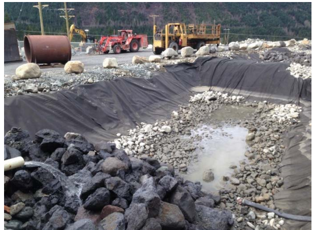
Photo 10 – BDRHEF powerhouse settling ponds; water infiltrating to ground in first cell (April 1, 2015).
