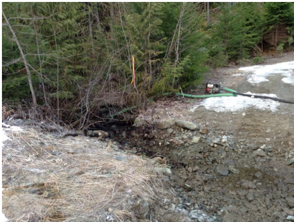
Photo 6 – Pump used to complete worksite isolation for culvert installation at MB47 on the Miller Bench FSR (March 17, 2015).
