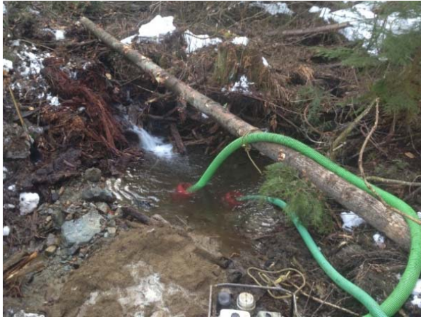
Photo 1 – Two pumps used to complete worksite isolation for culvert installation at 2+700 on road 197.2 (March 10, 2015).
