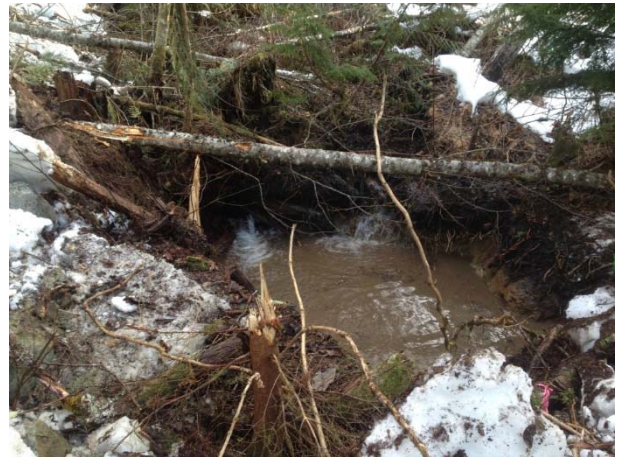
Photo 4 – Sump excavated to allow water to be pumped for worksite isolation during culvert installation at 1+335 on road 197.2 (March 4, 2015).
