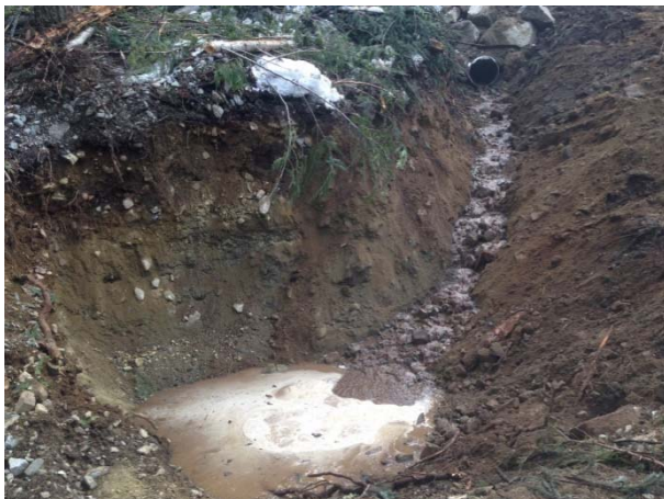
Photo 5 – Settling pond used to improve water quality following culvert installation on access road at 1+890 on road 197.2 (March 5, 2015).
