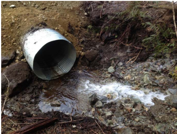
Photo 3 – A temporary pulse of suspended sediment was observed when water was released through new culvert at 1+911 on road 197.2 (March 3, 2015).
