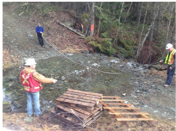
Photo 8 – Pre-work meeting discussing temporary clear span crossing upgrades at 1 of 3 crossing locations on the Miller Bench FSR (February 26, 2015).
