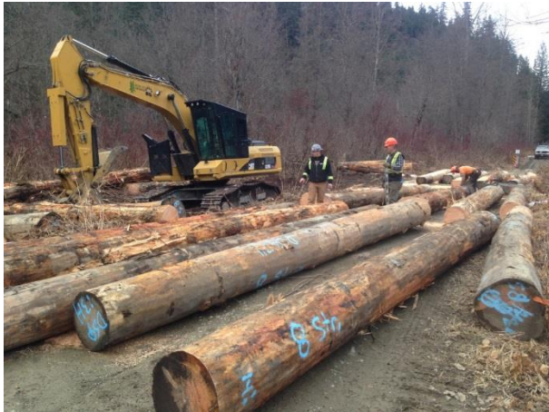
Photo 9 – Staging and preparing stringer and sill logs for the temporary log bridge structure to be installed on the Miller Bench FSR (February 26, 2015).
