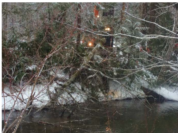
Photo 9 – Removing a tree from the Salmon Slough with ropes attached to an excavator (January 22, 2015).
