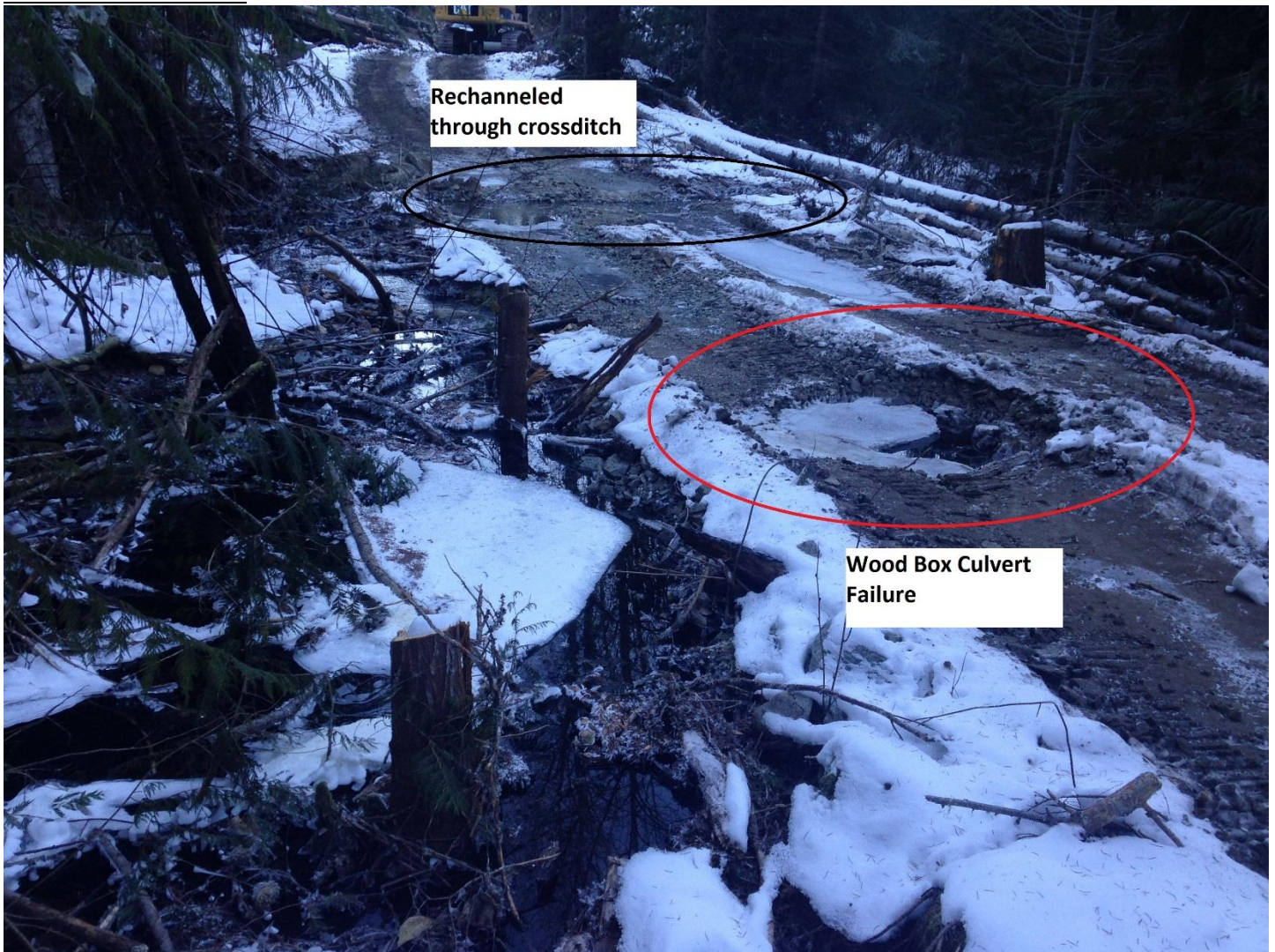
Collapsed WBC in foreground, cross-ditch in background.
