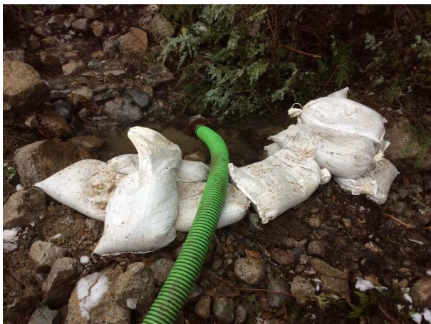
Photo 6 – Example of a sand bag berm and pump diversion installed to divert water around the work area during culvert installations along the Salmon main road (December 19, 2014).
