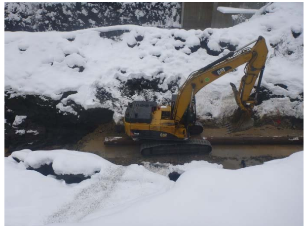
Photo 8 – Culvert installation being completed during the installation of the downstream cofferdam (November 26, 2014).
