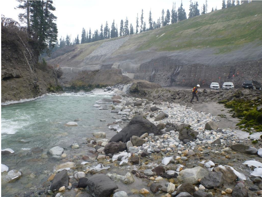
Figure 1. View downstream to intake cofferdam site. Temporary diversion channel is located at right of image.
