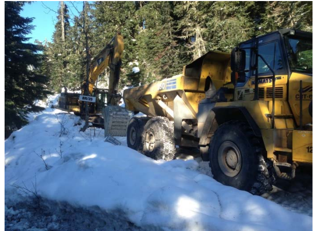
Photo 12 – Staging equipment in preparation for demobilization through the Mountain Goat Migration Corridor (November 29, 2014)
