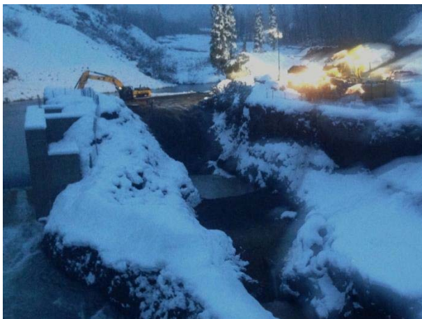
Photo 9 – Raising the height of the upstream cofferdam following completion of the downstream cofferdam works (November 26, 2014).
