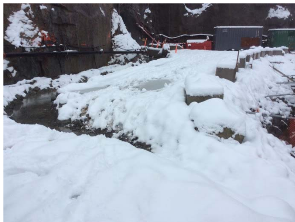
Photo 17 – A cut-off ditch installed to direct seepage from the tunnel excavation to the powerhouse excavation (November 26, 2014).
