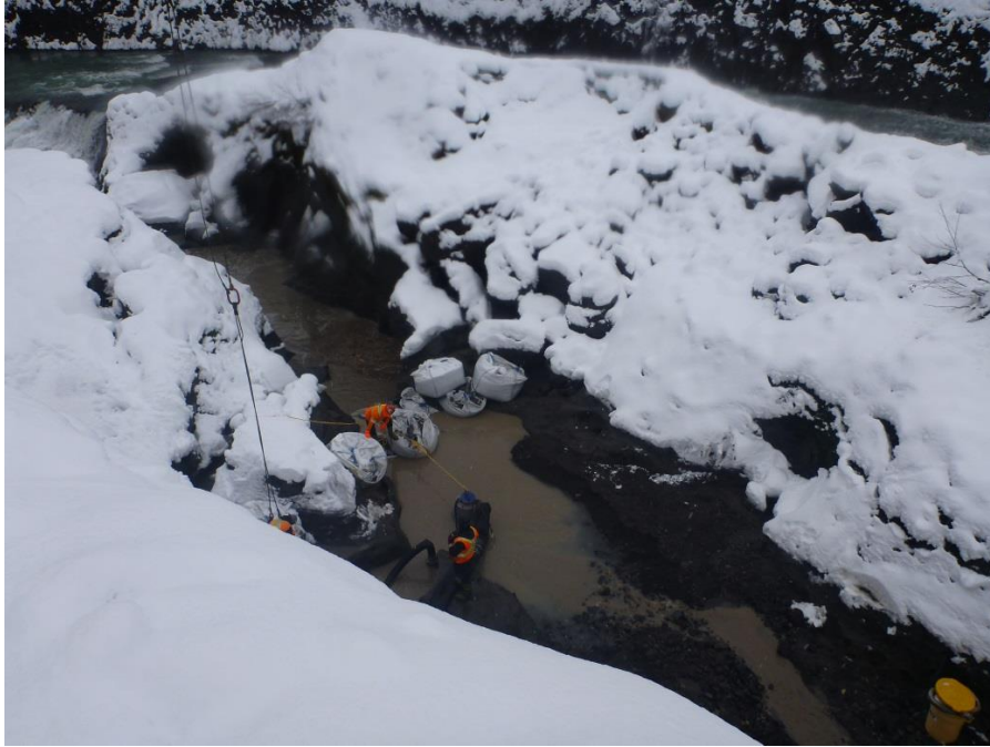
Figure 3. View of the large bags of clear-crush stone used to create a settlement pond downstream of the upstream cofferdam, which effectively slowed flows during the installation of fine material and allowed for deposition.
