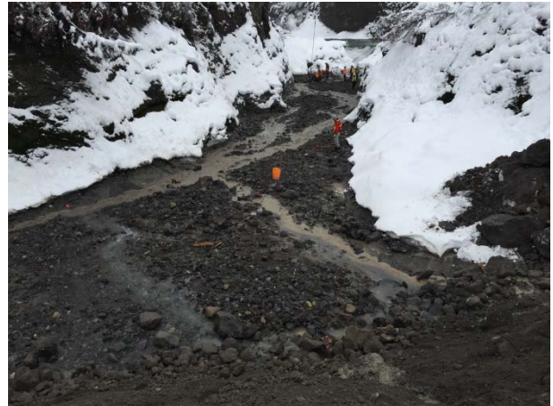
Photo 6 – Looking downstream at the diversion reach during the fish salvage works once the 0-300mm material sealed the majority of seepage (November 25, 2014).
