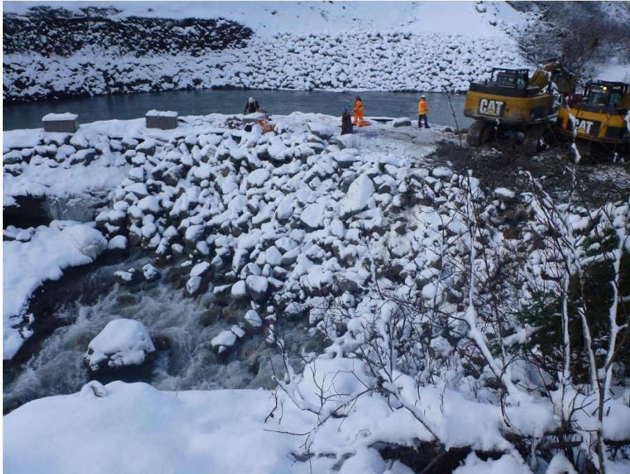
Figure 11. Additional rock fill material was placed on the toe of the cofferdam to seal the geomembrane to the base.
