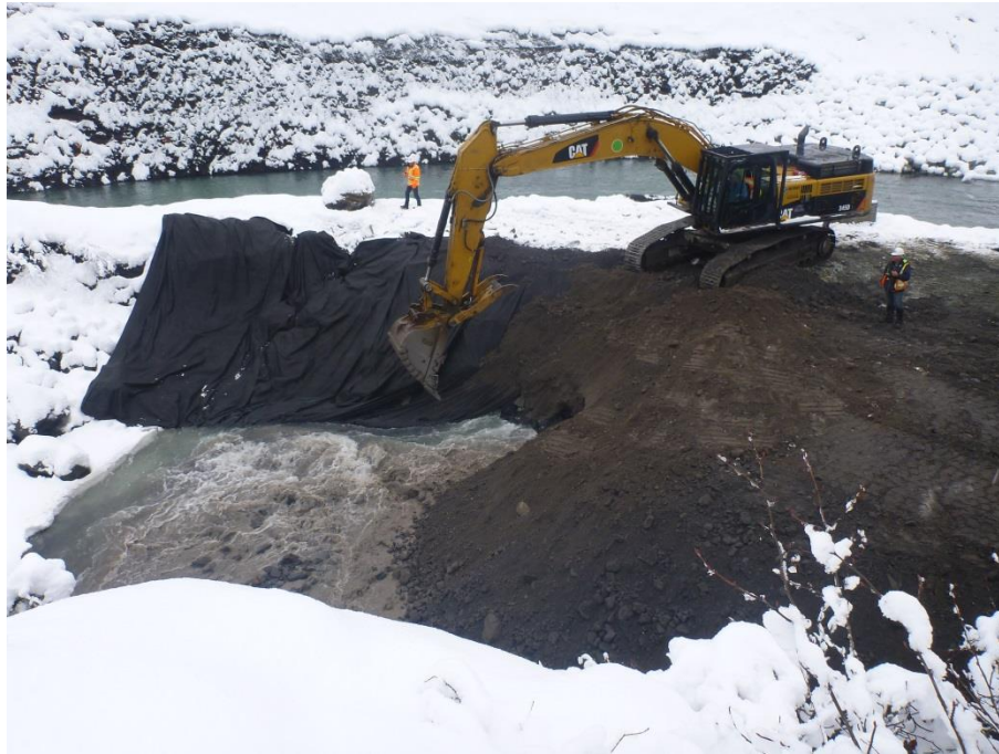
Figure 19. As works progressed across the channel fine material was sloughing out from the bottom of the cofferdam, requiring fast work and additional material.
