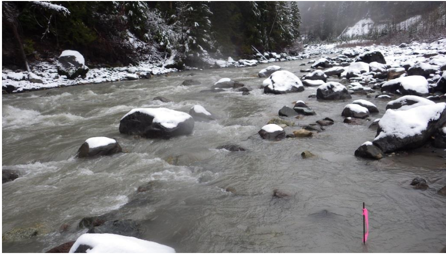
Figure 54. Elevated turbidity at site DSSD03 during infill of fine material at the cofferdam upstream.
