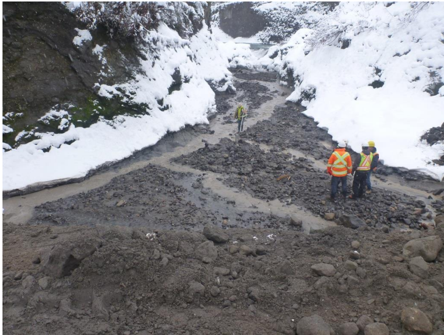
Figure 21. View downstream from the top of the cofferdam along the dewatered natural river channel. Small volumes of seepage are visible from the right and left corners of the cofferdam.
