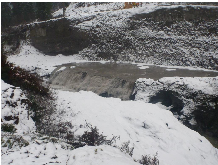
Figure 6. The initial flooding of the temporary diversion channel resulted in a significant flush of suspended sediment and turbidity which coincided with the flow stage change induced during the switch.
