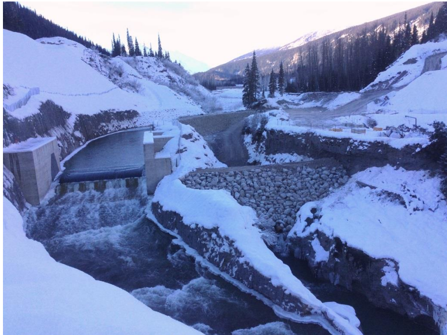
Figure 29. View of the completed cofferdams and dewatered river channel to the right of the image. The flows were successfully diverted through the temporary diversion channel, with the Obermeyer in place, to the left of the image.
