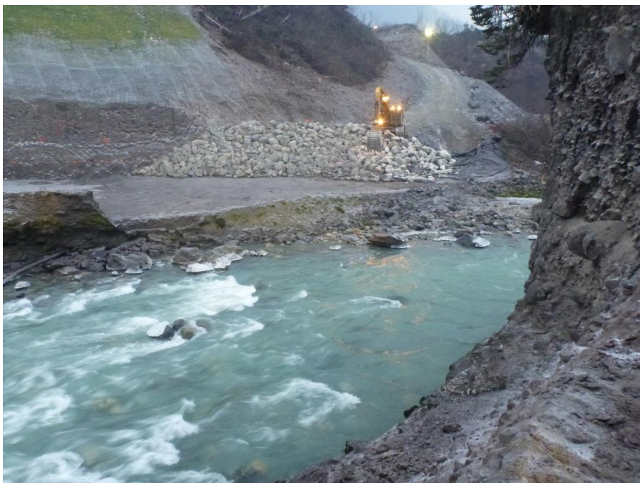
Figure 2. Rock armour placement at right bank of temporary diversion channel. View from river-left.
