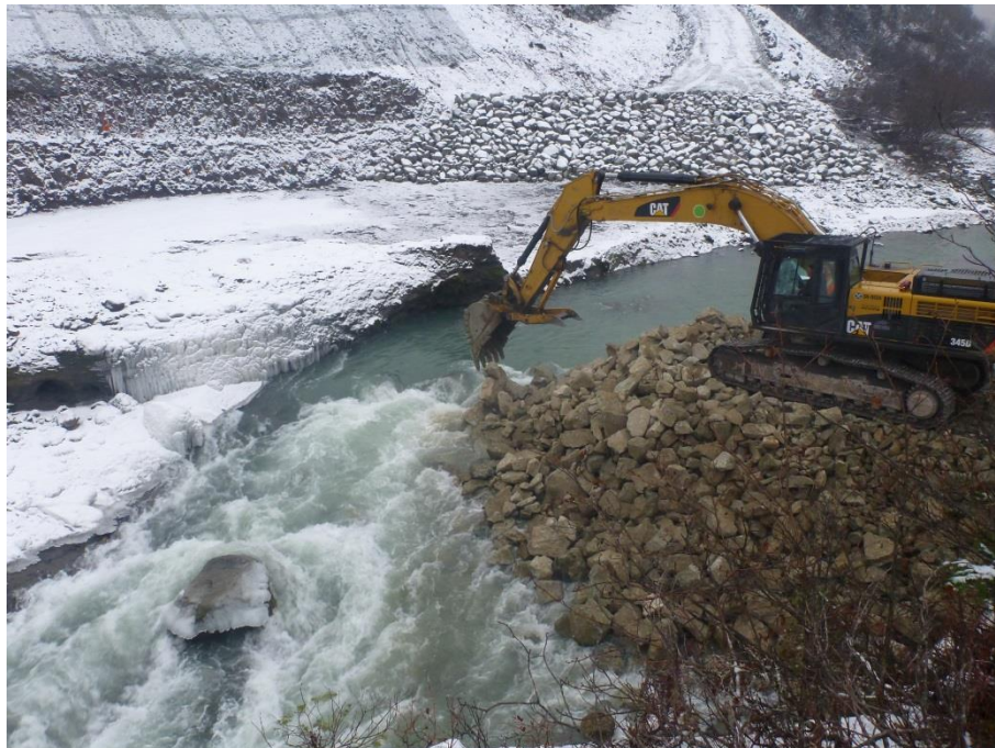
Figure 4. Building out first rock layer of cofferdam across the river channel. Water level rising upstream.
