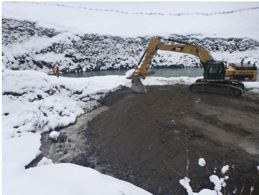
Figure 20. The flows through the cofferdam were sealed with the last section of fine material completed.
