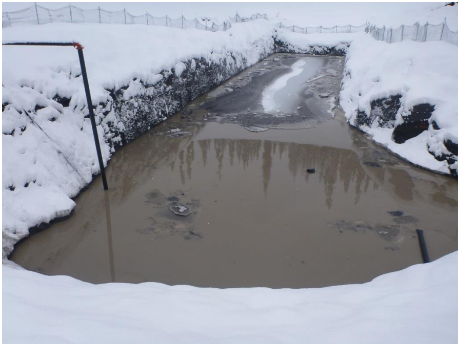
Figure 4. View of the upstream tunnel portal excavation into which sediment-laden water was pumped from the temporary settlement pond downstream of the upstream cofferdam.
