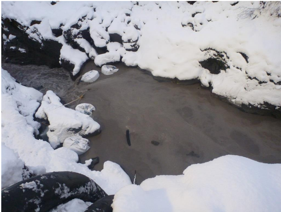
Figure 17. Large bags of crushed stone were in place downstream of the cofferdam to create a check in flow velocities. Two pumps were pumping out water to the upstream tunnel portal excavation.
