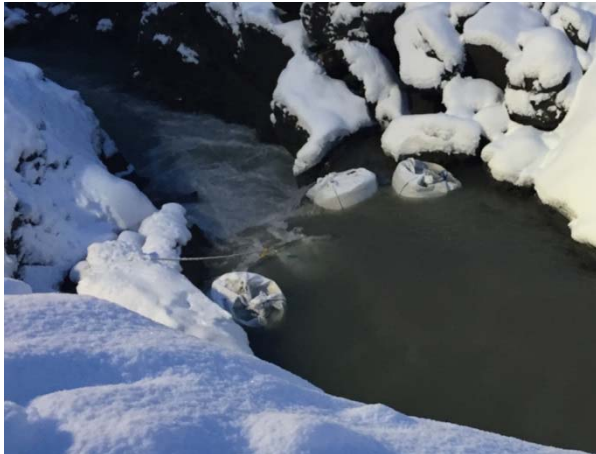
Photo 5 – One ton bags filled with crushed rock installed downstream of the cofferdam to create a sediment trap (November 25, 2014).
