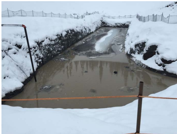
Photo 7 – ULRHEF upstream tunnel portion excavation filled with sediment laden water that was pumped during the cofferdam installation works. (November 25, 2014).
