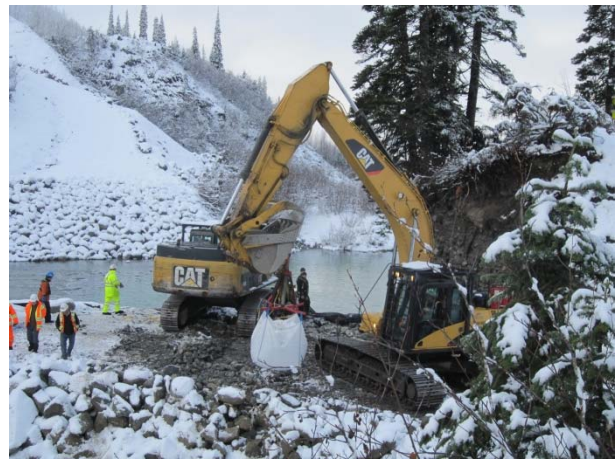
Photo 2 – Placing 1 ton bags of crushed rock on the upstream side of the cofferdam (November 23, 2014)
