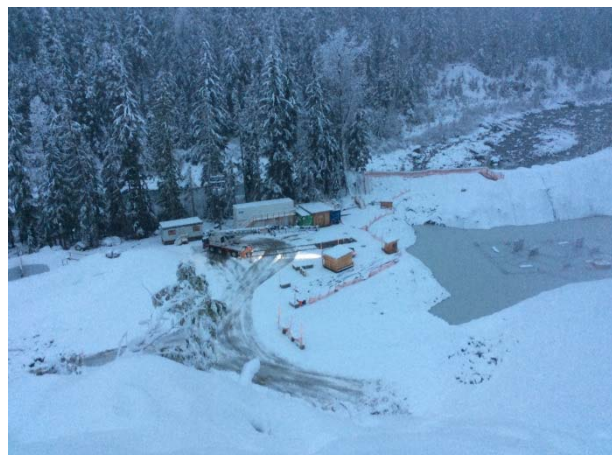
Photo 13 – Final demobilization from the ULRHEF powerhouse site. Note the flooded powerhouse area. (November 26, 2014).
