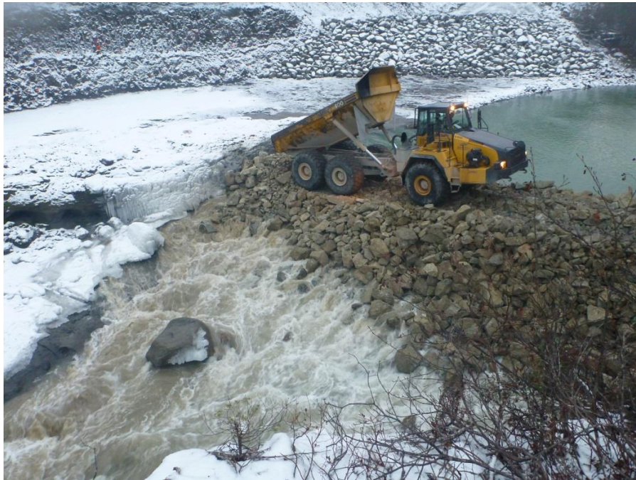
Figure 5. Closing the first rock layer across the river channel. This induced a significant rise in water level upstream, reaching the temporary diversion channel and switching flows.
