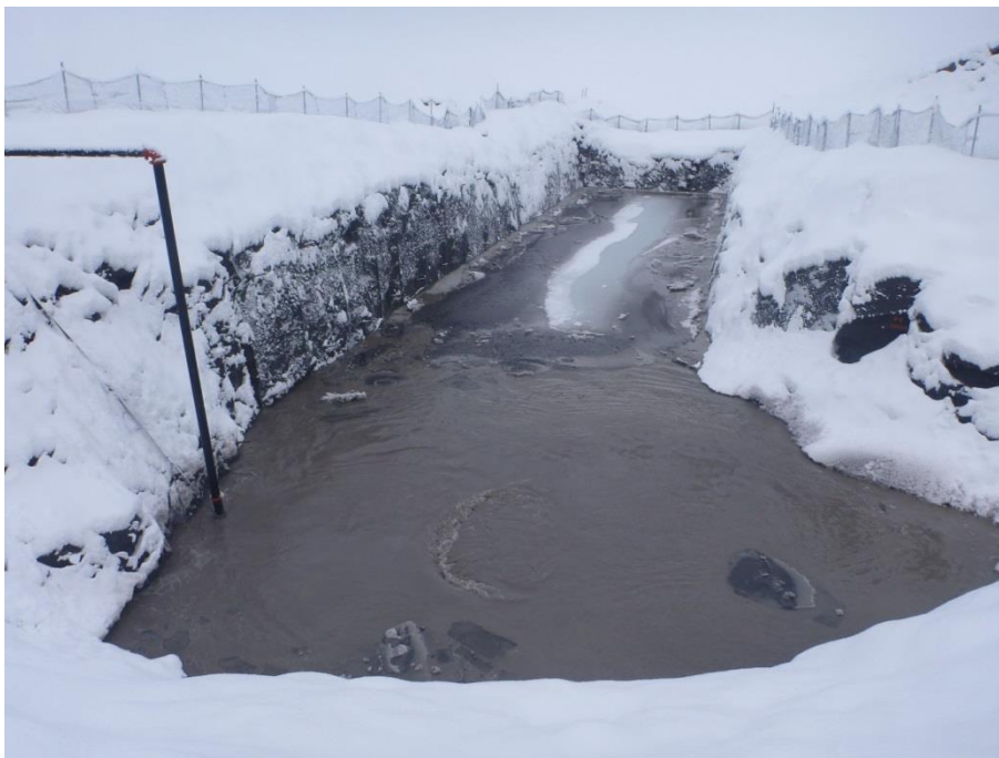
Figure 18. View of the upstream tunnel portal excavation settlement pond filling with turbid water from the river channel.
