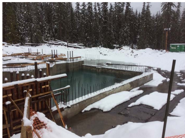
Photo 16 – Flooded BDRHEF powerhouse area following demobilization of dewatering equipment. (November 26, 2014).
