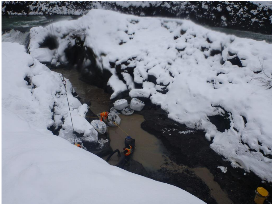
Figure 22. Using the crane the pumps were removed from the channel downstream. The volume of coarse sand, gravel and fines that had deposited here illustrates the success of this mitigation measure.
