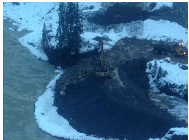
Photo 10 – Placement of riprap armouring on the front face of the upstream cofferdam once it was built to design height (November 27, 2014).
