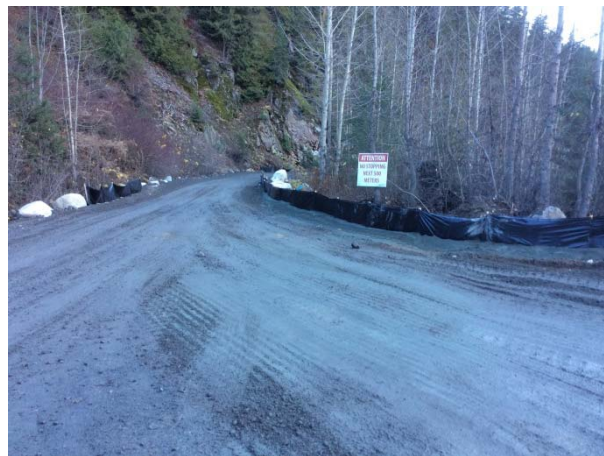
Photo 24 – Silt fencing repaired and installed from KM 41 to KM 42 on the Lillooet River FSR (November 10, 2014).
