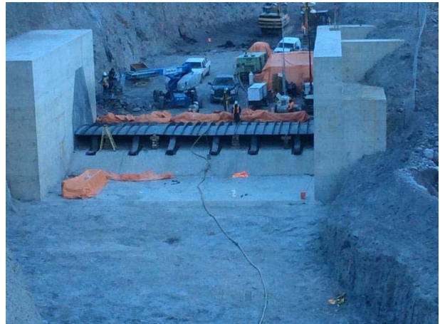
Photo 2 – Installation of final Obermeyer Weir components at the ULRHEF intake diversion channel (November 15, 2014).
