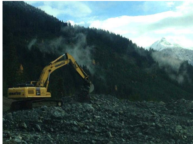
Photo 12– Re-grading of PAG stockpile at KM 44.5 on the Lillooet River FSR (November 9, 2014).
