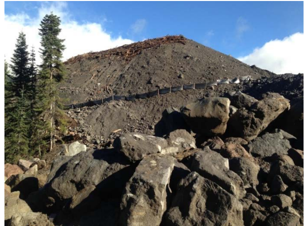
Photo 8 – Silt fencing installed midway up slope on north side spoil pile (November 10, 2014).
