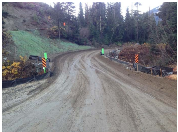
Photo 10 – Silt fencing installed and road grading completed at the KM 48 box culvert (November 7, 2014).
