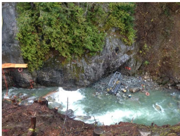
Photo 37 – Ecofish crew conducts Coastal Tailed Frog salvage downstream of BDRHEF intake diversion tunnel site (November 4, 2014).
