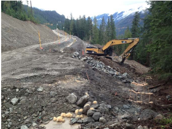
Photo 21 – Stabilization works and erosion and sediment control measures at 2+800 fill slope (November 8, 2014).
