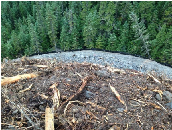
Photo 7 – Silt fence installed at toe of slope and organic material placed on north side spoil pile (November 8, 2014).
