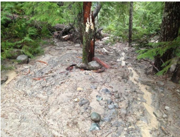
Photo 19 – Material mobilizing beyond project boundaries below toe of 2+800 fill slope (November 3, 2014).
