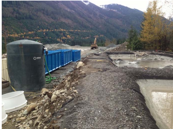
Photo 40 – Active water treatment system installed at BDRHEF portal settling ponds (November 8, 2014).
