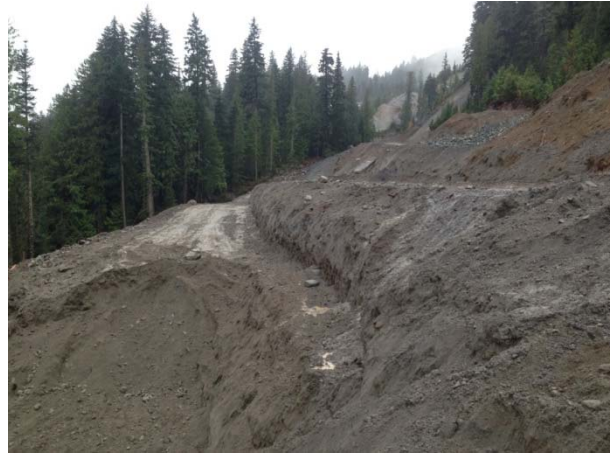
Photo 18 – Sloughing and failures observed at station 2+800 fill slope (November 3, 2014).
