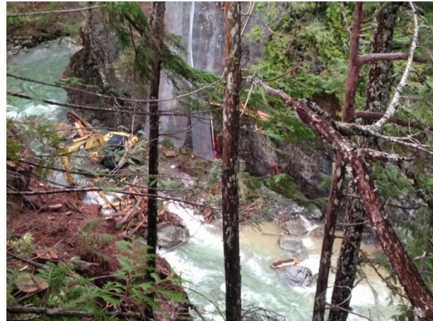
Photo 30 – Excavator used for log jam removal; sediment plume visible downstream of works (November 4, 2014).
