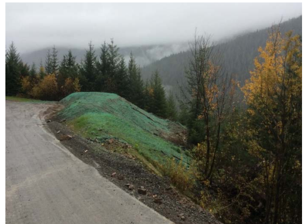
Photo 16 – Re-contouring of failing material at KM 43.5 on the Lillooet River FSR (November 3, 2014).
