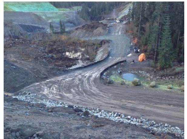
Photo 8 – Silt fencing installed around tributary and ditching completed on ULRHEF intake south side access road (November 7, 2014).
