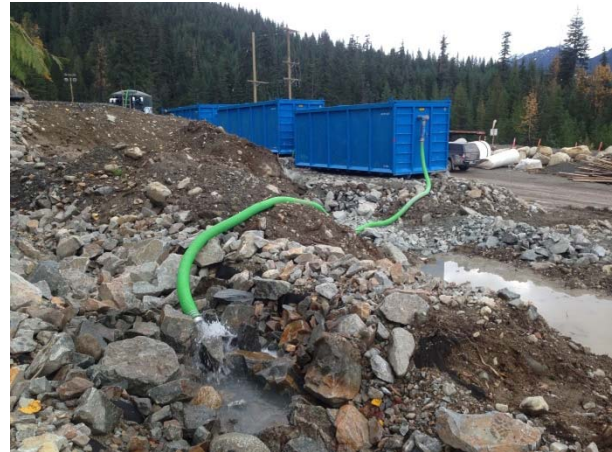
Photo 41 – Active water treatment system activated at BDRHEF portal settling ponds (November 8, 2014).
