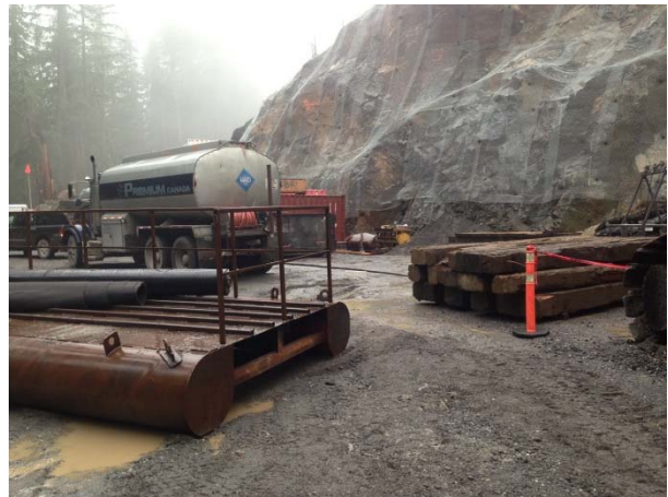
Photo 32 – Platforms cleaned on crane pad prior to being installed at diversion tunnel site (November 5, 2014).
