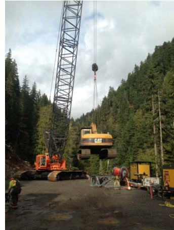
Photo 28 – CAT 320 excavator lifted with crane and mobilized to left bank for diversion tunnel works (November 4, 2014).
