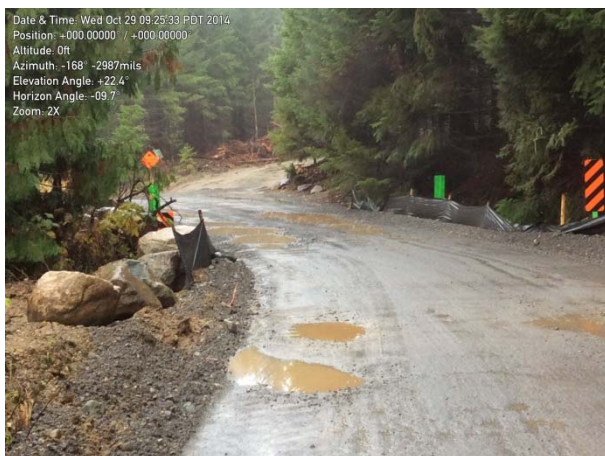
Photo 28 – Box culvert at KM 39.7 on the Upper Lillooet FSR; sediment fencing requires repair (October 29, 2014).
