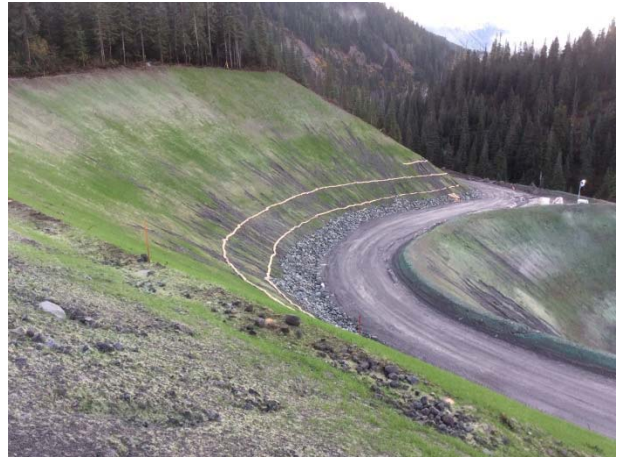
Photo 6 – Curlex sediment logs installed on north side access road slope; sediment logs will reduce rill erosion and mobilization of sediment (October 31, 2014).
