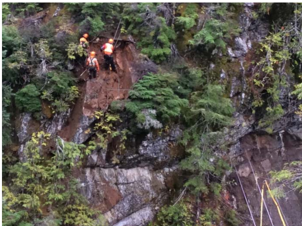
Photo 24 – Rope access crews conduct scaling works on left bank at BDRHEF intake (October 30, 2014).
