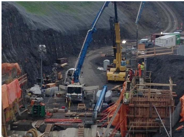
Photo 4 – ULRHEF intake diversion channel Obermeyer weir concrete works (Obermeyer left walls) (October 26, 2014).
