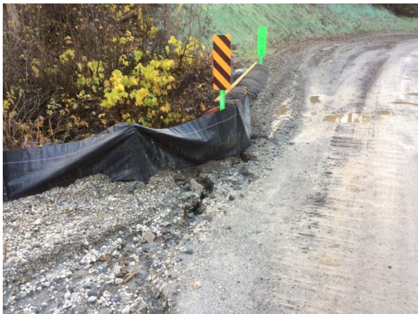
Photo 7 – Failing silt fence and rilling on road at KM 48 box culvert (October 31, 2014).
