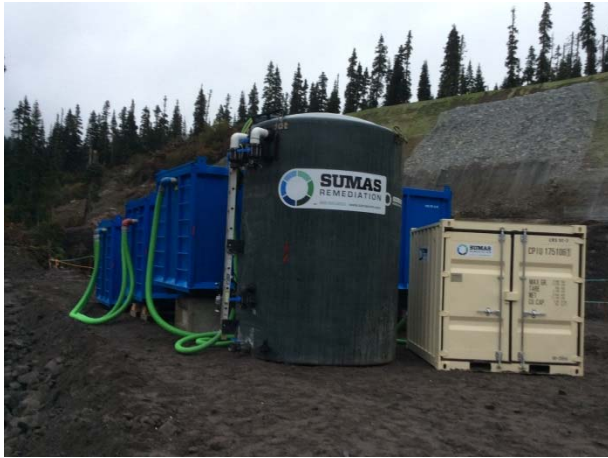
Photo 5 – Active water treatment system installed to dewater ULRHEF upstream portal excavation (October 27, 2014).
