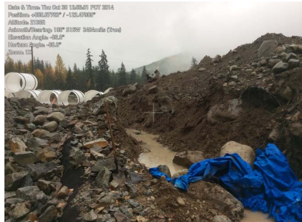
Photo 27 – Turbid seepage discharging from below BDRHEF downstream tunnel portal sediment pond (October 30, 2014).
