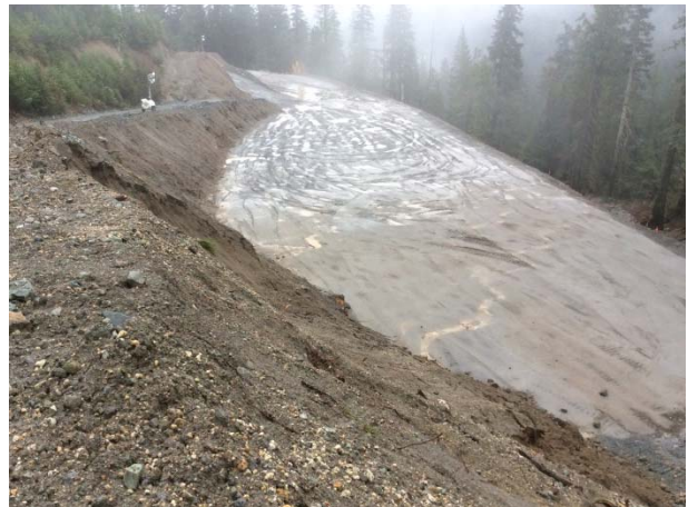
Photo 15 – Conditions at 2+800 fill slope during significant rain event (October 31, 2014).
