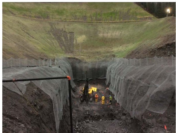
Photo 2 – Excavation continued, including drilling and blasting, at the ULRHEF upstream tunnel portal (October 27, 2014).
