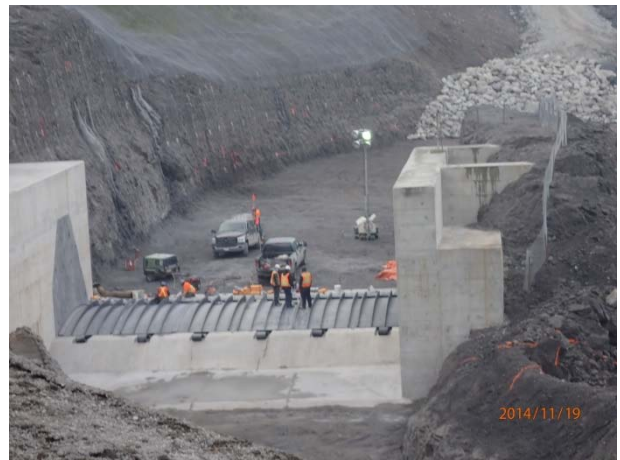
Photo 6 – Final testing of the Obermeyer weir (November 19, 2014).
