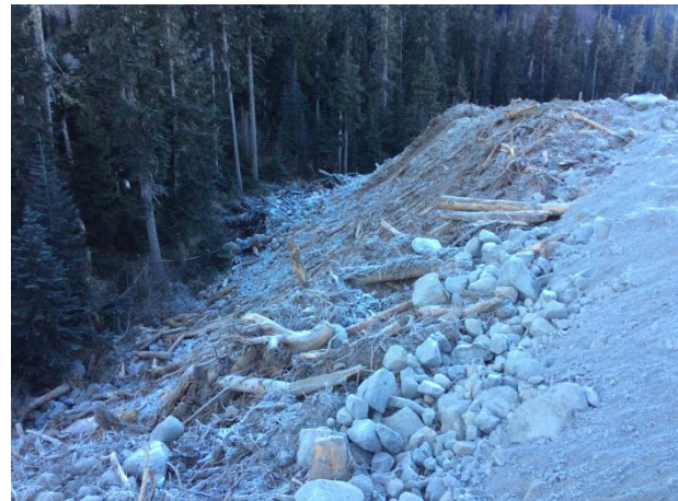
Photo 2 – Slopes of the south side spoil area at the ULRHEF intake have been shaped and covered with organic material (November 16, 2014).
