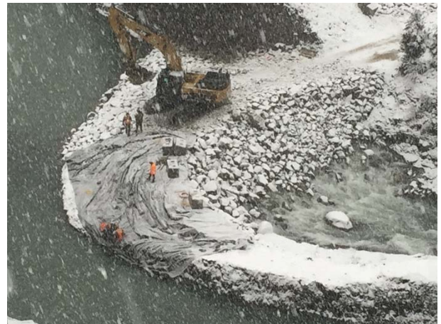
Photo 10 – Placement of the geo-membrane on the front face of the cofferdam (November 21, 2014).
