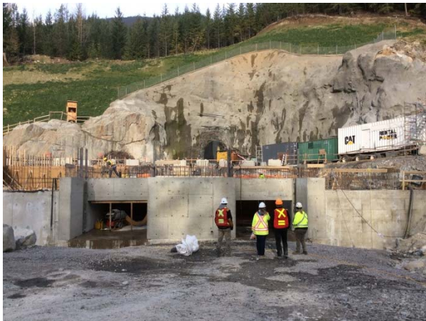
Photo 17 – Current conditions at BDRHEF powerhouse, continued rebar/formworks and concrete structure pour (November 17, 2014).
