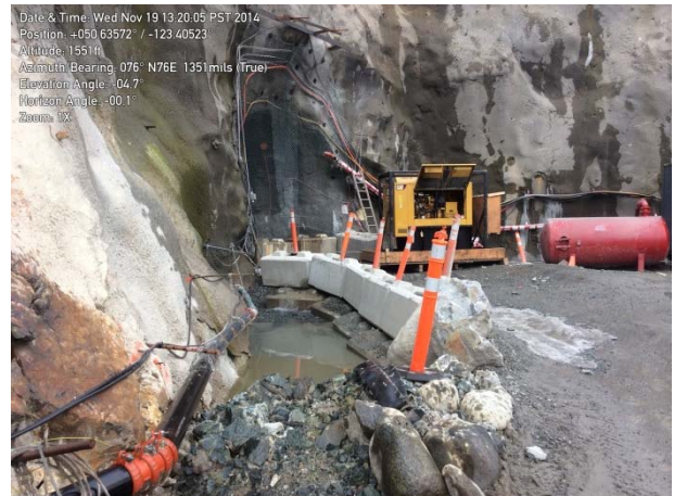
Photo 18 – BDRHEF downstream tunnel portal with wire mesh installed to prevent access (November 19, 2014).
