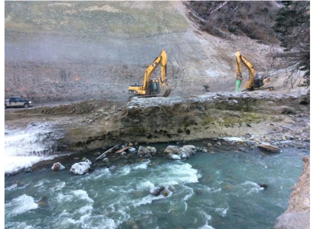
Photo 4 – ULRHEF intake diversion channel upstream plug excavation. No work occurred instream (November 16, 2014).
