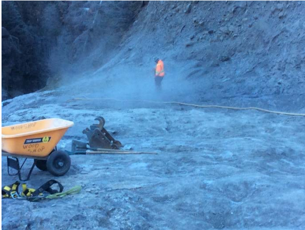
Photo 3 – Cleaning of the diversion channel with pressurized air and collection of the material with hand tools (November 16, 2014).
