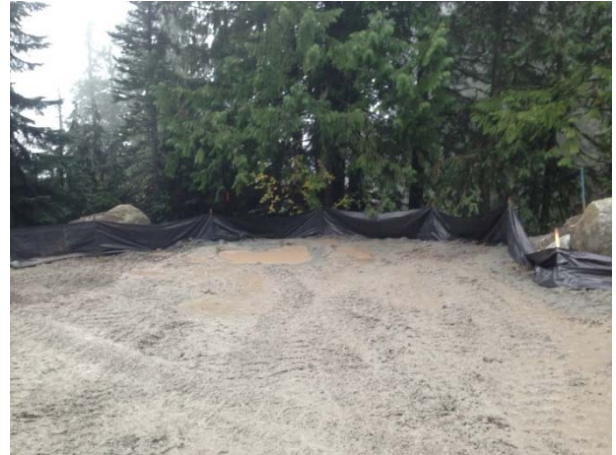
Photo 12 – Sediment fencing around perimeter of rock truck turn-around area located at station 2+660 (October 19, 2014).
