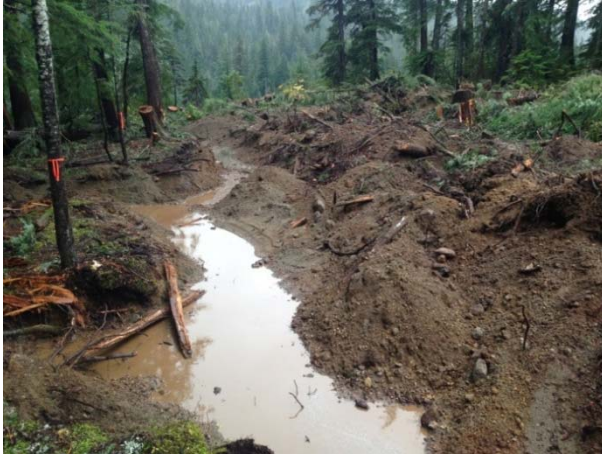
Photo 15 – Drain installed at 3+875; water was observed infiltrating to ground during significant rain event (October 22, 2014).
