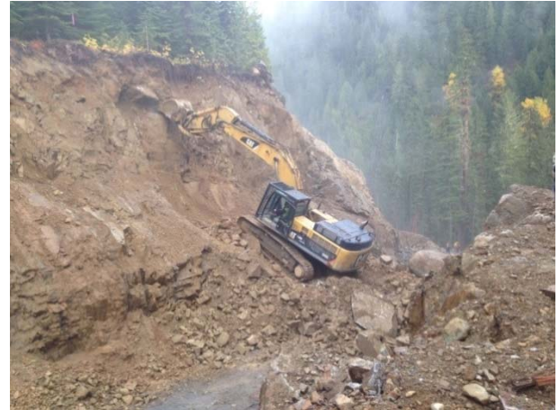
Photo 19 – Continued scaling works following rock fall at KM 4.75 on BDRHEF intake access road (October 22, 2014).
