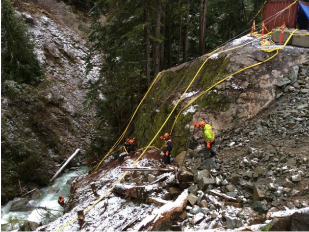
Photo 22 – Rope access crew conduct rock bolt stabilization works on the right bank at BDRHEF intake (October 25, 2014).
