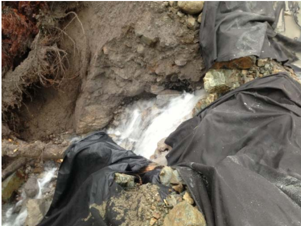
Photo 5 – Failure at north side settling pond spillway (October 20, 2014).
