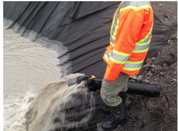
Photo 4 – A flocculant sock was applied to inlet of north side settling pond for water treatment (October 19, 2014).
