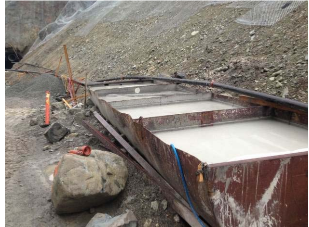
Photo 10 – ULRHEF downstream portal oil water separator (October 19, 2014).
