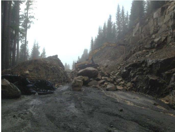
Photo 18 – Scaling works following rock fall at KM 4.75 on BDRHEF intake access road (October 22, 2014).
