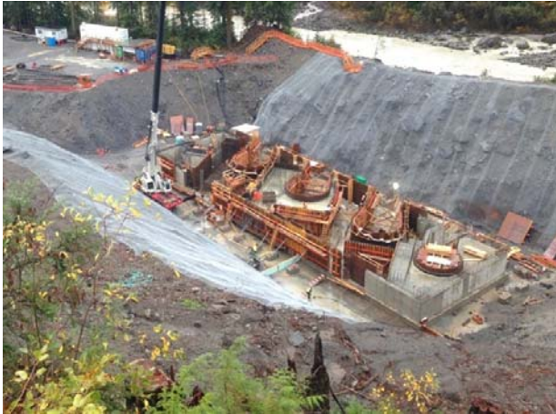
Photo 17 – Current conditions at ULRHEF powerhouse; rebar and formworks continued during this reporting period (October 22, 2014).
