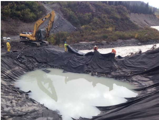
Photo 7 – ULRHEF intake north side settling pond repair works in progress; replacement geotextile liner was installed (October 20, 2014).
