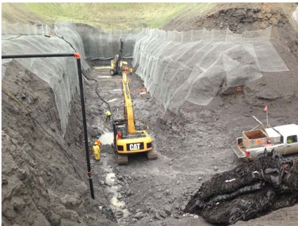
Photo 1 – Bulk excavation, including drilling and blasting, continued at the upstream tunnel portal (October 19, 2014).
