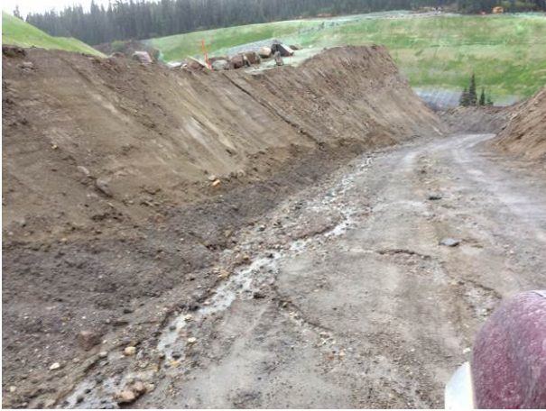
Photo 5 – ULRHEF intake north side cofferdam access road, ditching requires attention (October 14, 2104).
