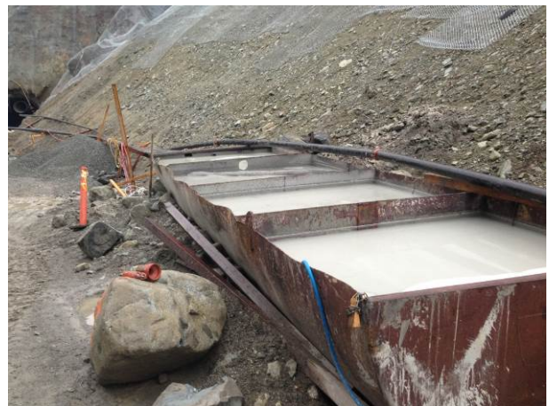
Photo 9 – ULRHEF downstream portal oil water separator (October 16, 2014)
