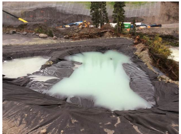
Photo 4 – ULRHEF intake north side settling pond adjacent to cofferdam access road (October 14, 2014).
