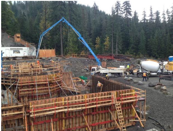
Photo 19 – Current conditions at BDRHEF powerhouse, continued rebar/formworks and concrete structure pour (October 16, 2014).
