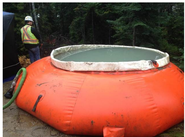
Photo 11 – Water bladder for ULRHEF tunnel exploratory borehole drilling at KM 46.5 on the Lillooet River FSR (October 16, 2014).
