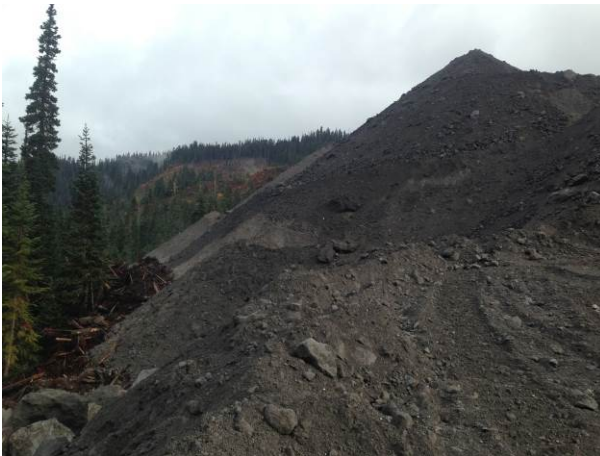
Photo 7 – ULRHEF intake spoil are (north side) requiring additional mitigation prior to winter shutdown (October 16, 2014).
