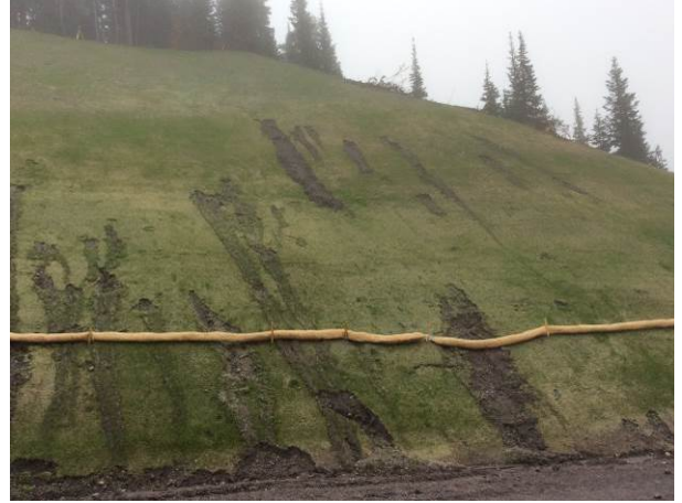
Photo 6 – ULRHEF intake north side cut slopes with hydroseed and initial Curlex log installation, requires further attention (October 14, 2014).
