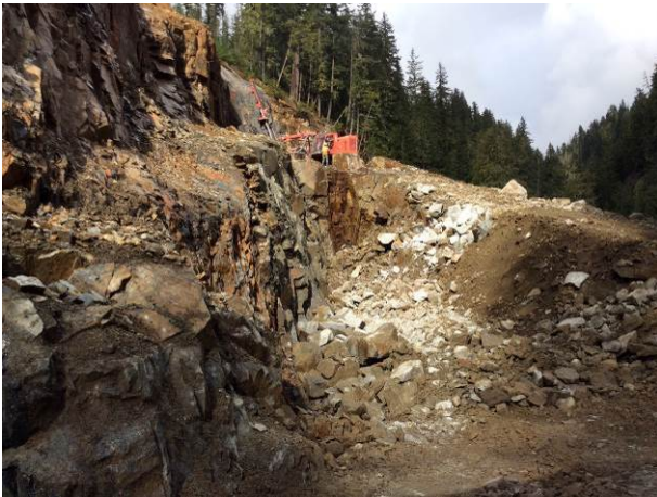
Photo 17 – BDRHEF crane pad excavation and drilling/blasting at top level of crane pad (October 14, 2014).
