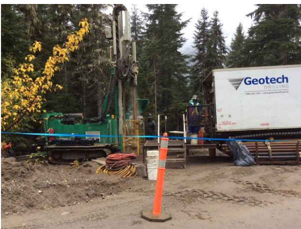
Photo 10 – ULRHEF tunnel exploratory borehole drilling at KM 46.5 on the Lillooet River FSR (October 15, 2014).
