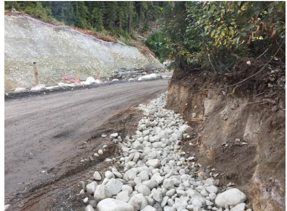
Photo 10 – French drain installation of ULRHEF downstream tunnel portal access road completed on the woods side (October 9, 2014).
