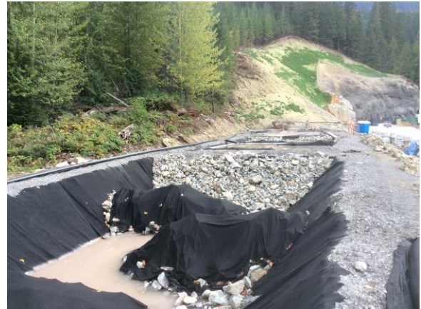
Photo 20 – BDRHEF powerhouse settling pond, no discharge observed; however pond #1 remains full of sediment and requires maintenance (September 30, 2014).
