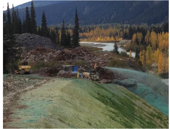
Photo 6 – Hydroseeding and drainage ditch works above the south side cut slope at ULRHEF intake (October 7, 2014).
