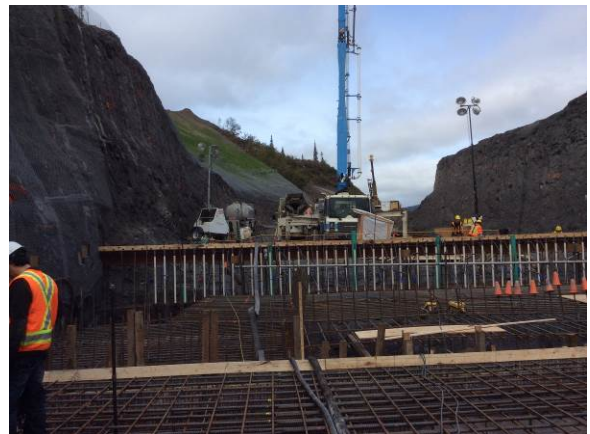
Photo 4 – Obermeyer weir structure pour, alkaline water was treated with CO 2 injection as required system prior to discharge (October 5, 2014).
