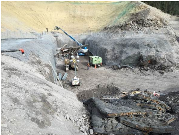
Photo 1 – Overview of wire mesh and rock anchor installation at the north side of the ULRHEF intake (October 9, 2014).
