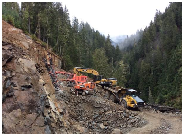
Photo 17 – BDRHEF crane pad excavation and drilling/blasting at top level of crane pad (October 11, 2014).
