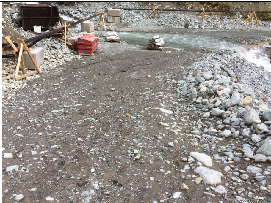
Photo 10. The ULRHEF lower tunnel portal access road drainage discharges directly to Truckwash Creek. Ditch improvements and road grading is required to protect surface water quality.
