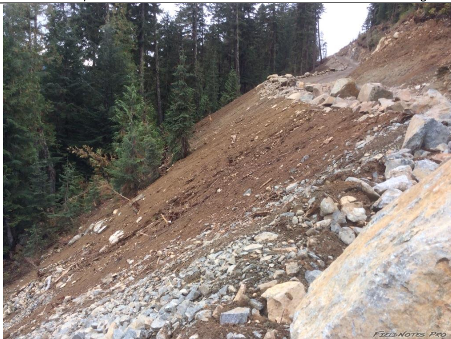
Photo 12. Newly contoured/completed slopes along the BDRHEF intake access road required erosion protection (example 1)
