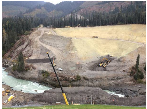
Photo 8 – ULRHEF north side drilling/blasting for tunnel portal bulk excavation and construction of settling pond (October 3, 2014).
