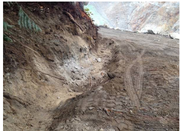
Photo 12 – French drain installation of ULRHEF downstream tunnel portal access road, woods side (October 1, 2014).
