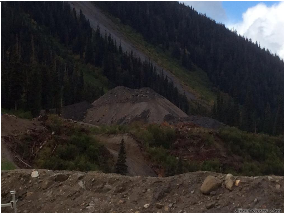
Photo 4. The south spoil area at the ULRHEF intake requires material consolidation, erosion protection and drainage installation to prevent further erosion and the generation of sediment laden runoff. Recommend contouring to final design slopes, capping final slopes with organic material and hydro-seeding as a temporary ESC protection measure (with slope appropriate mulch type), until the final reclamation prescription is presented and approved.
