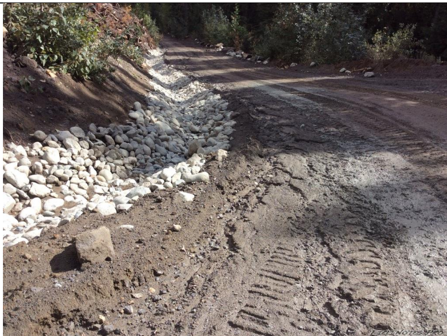
Photo 7. Ditches are not collecting and transporting road runoff as intended due to the road grading along the lower ULRHEF tunnel portal access road. Regrading of the road surface is recommended to direct runoff to the road side ditch and check dam installation is recommended to slow water velocities along the steep sections and permit sediments to drop out of suspension in the ditch line.
