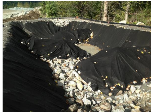
Photo 22 – BDRHEF powerhouse settling pond, no discharge observed; however pond #1 remains full of sediment and requires maintenance. (September 30, 2014).
