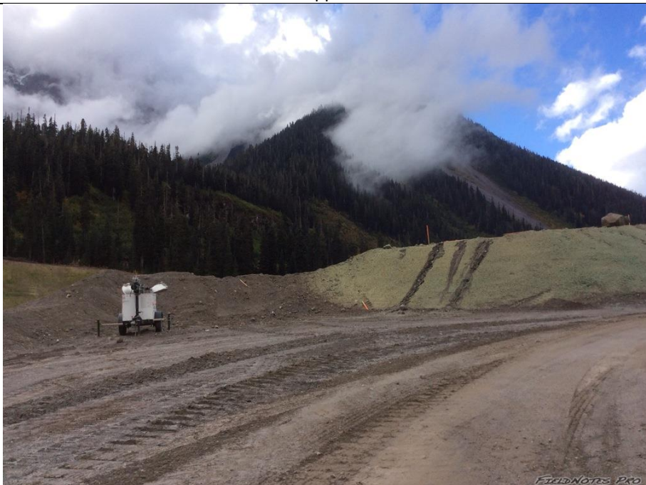
Photo 6. Rilling and gully erosion forming on the north side/upstream portal excavation cut slopes. The installation of velocity dissipation slope breaks to slow surface runoff or the application of a hydro-mulch better suited to the slopes (BFM or FGM) is recommended. Ditches should be cleaned and check dams installed/maintained as required. Erosion of the ditch line is not currently achieving intended ESC goals.
