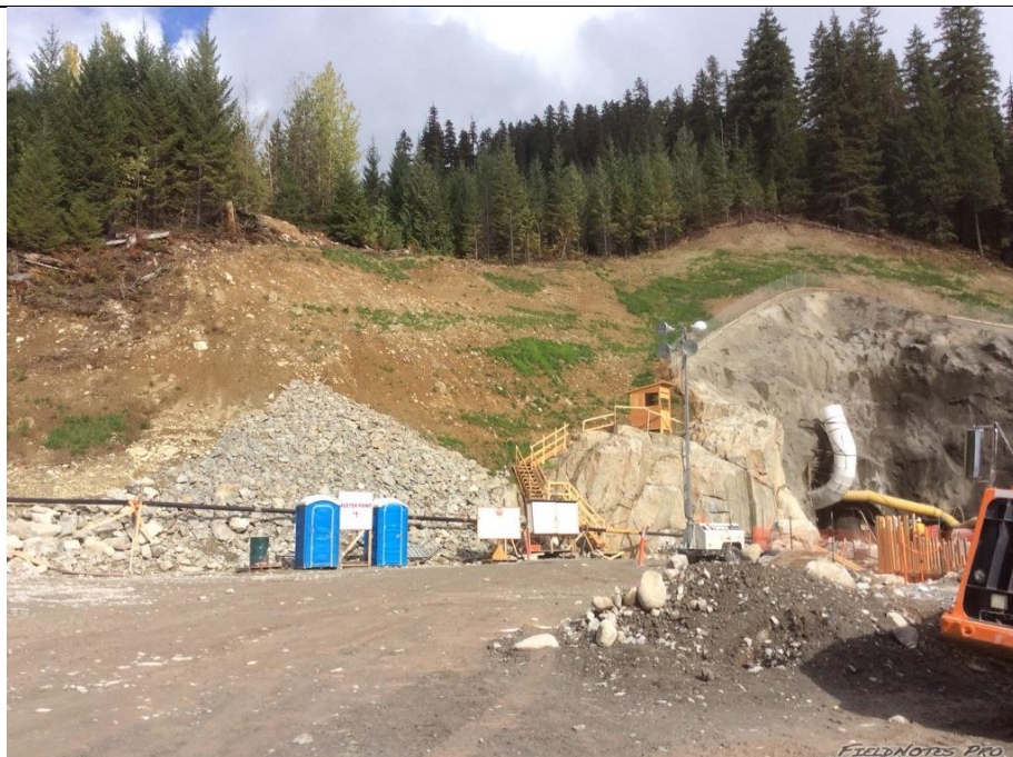
Photo 15. Slope stabilization measures required at the BDRHEF lower tunnel portal where hydro-seeding has been unsuccessful.
