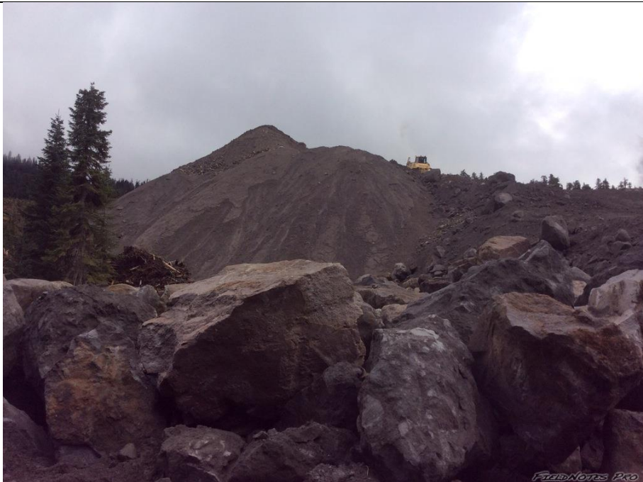
Photo 5. The north spoil area at the ULRHEF intake requires material consolidation, erosion protection and drainage installation to prevent further erosion and the generation of sediment laden runoff. Recommend contouring to final design slopes, capping final slopes with organic material and hydro-seeding as a temporary ESC protection measure (with slope appropriate mulch type), until the final reclamation prescription is presented and approved.
