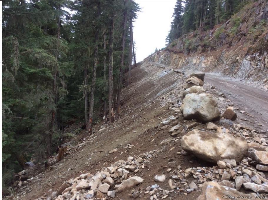
Photo 13. Newly contoured/completed slopes along the BDRHEF intake access road required erosion protection (example 2)
