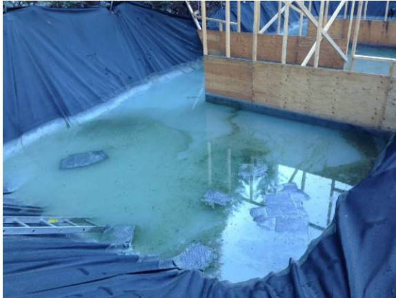
Photo 9 – ULRHEF downstream portal settling ponds following spill within tunnel, no discharge from ponds (September 28, 2014)
