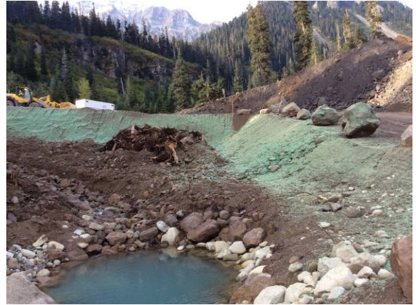
Photo 6 – Hydroseeding and drainage works near south side spoil area at ULRHEF intake (October 2, 2014).
