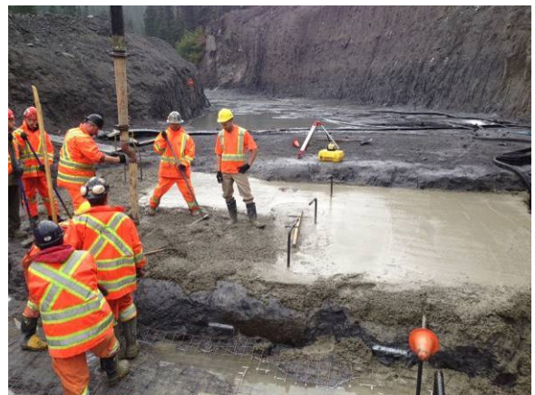
Photo 4 – Obermeyer weir mud slab pour, alkaline water was treated with CO 2 injection as required system prior to discharge (September 29, 2014).
