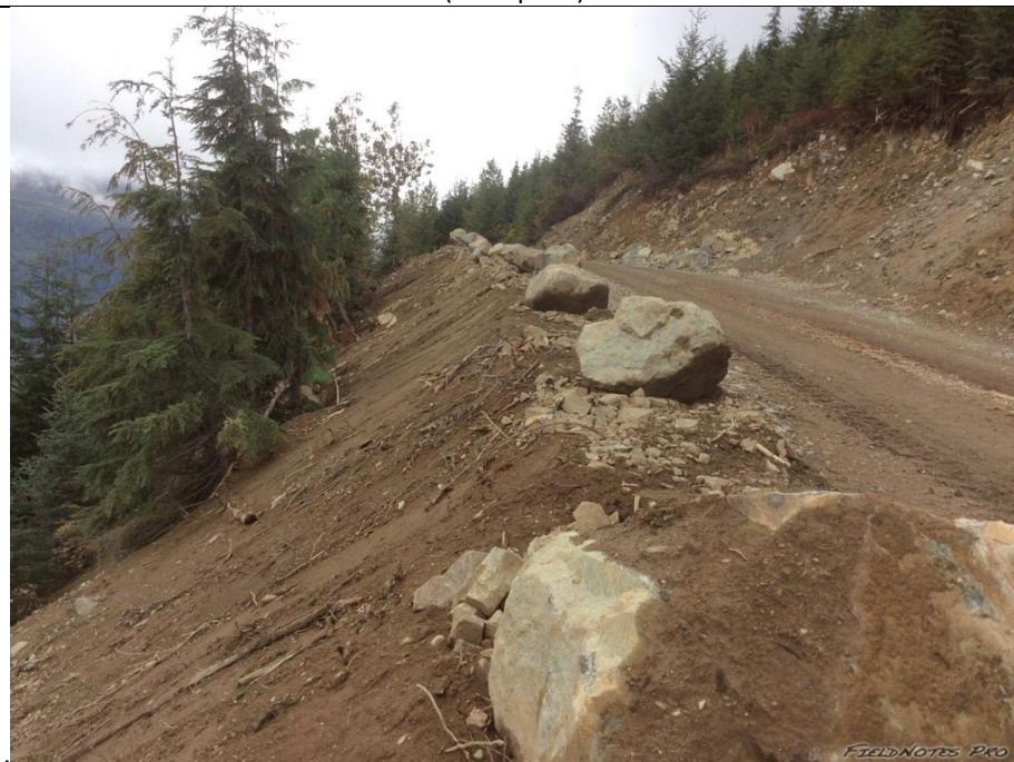
Photo 14. Newly contoured/completed slopes along the BDRHEF intake access road required erosion protection (example 3)
