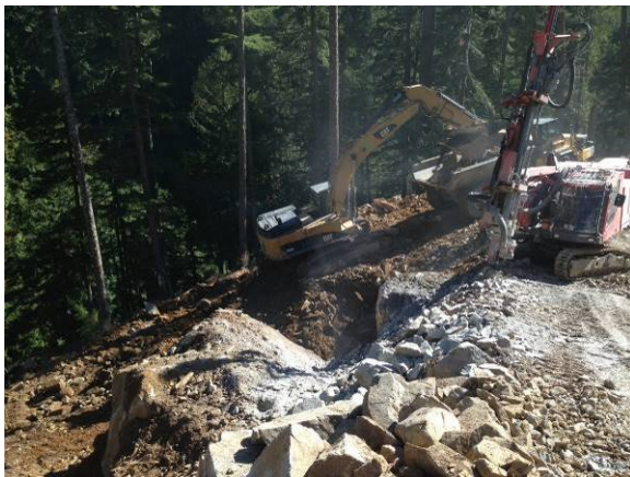
Photo 18 – BDRHEF crane pad excavation and drilling/blasting at top level of crane pad (September 28, 2014).
