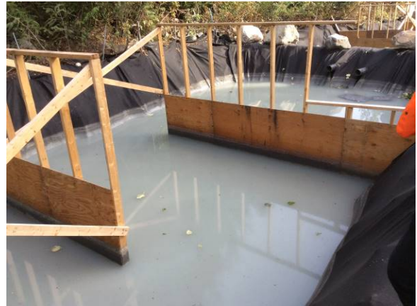
Photo 10 – ULRHEF downstream portal settling ponds following cleanup efforts, no visual or olfactory signs of hydrocarbons remained (October 2, 2014).
