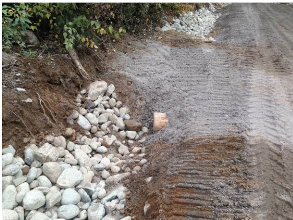
Photo 11 – ULRHEF downstream tunnel portal access road, drainage works included ditch block and culvert installation (October 1, 2014).
