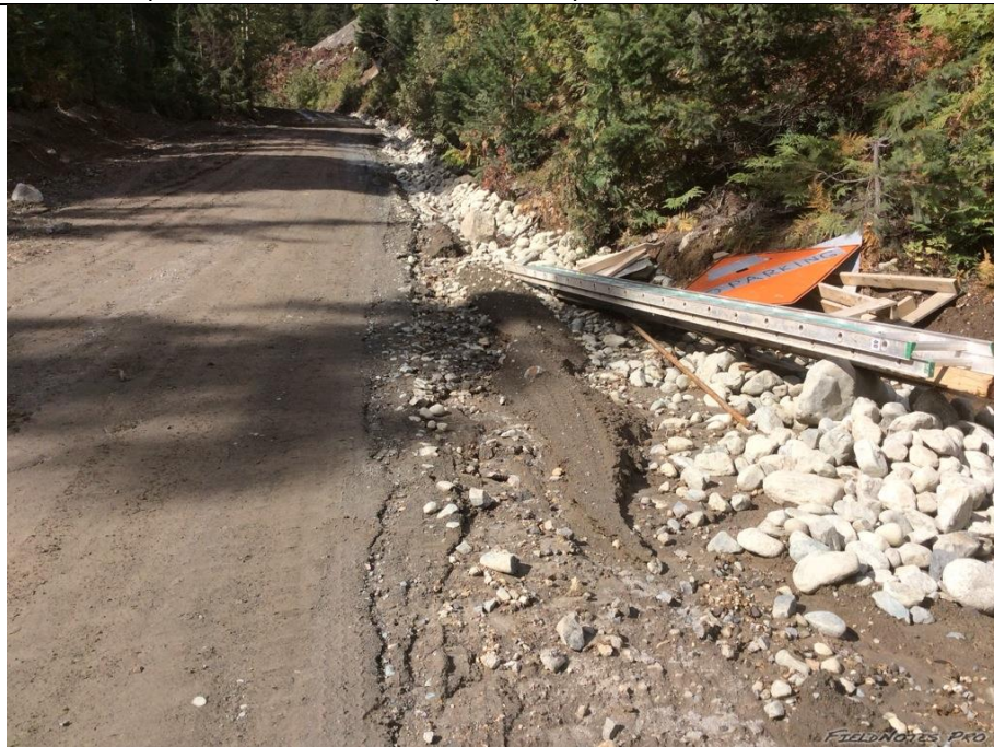
Photo 8. . Ditches are not collecting and transporting road runoff as intended due to the road grading along the lower ULRHEF tunnel portal access road. Regrading of the road surface is recommended to direct runoff to the road side ditch and check dam installation is recommended to slow water velocities along the steep sections and permit sediments to drop out of suspension in the ditch line.
