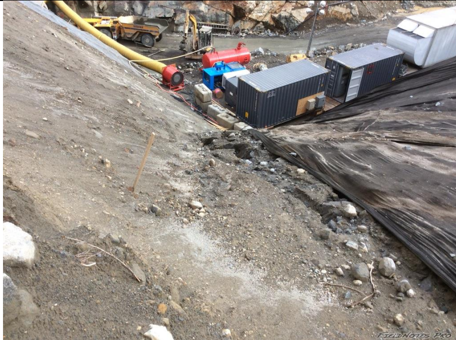
Photo 9. Gully erosion forming where road runoff flows over the edge of the slope into the ULRHEF lower portal work area. Directing road runoff away from this slope and installing slope protection to prevent further erosion is recommended.
