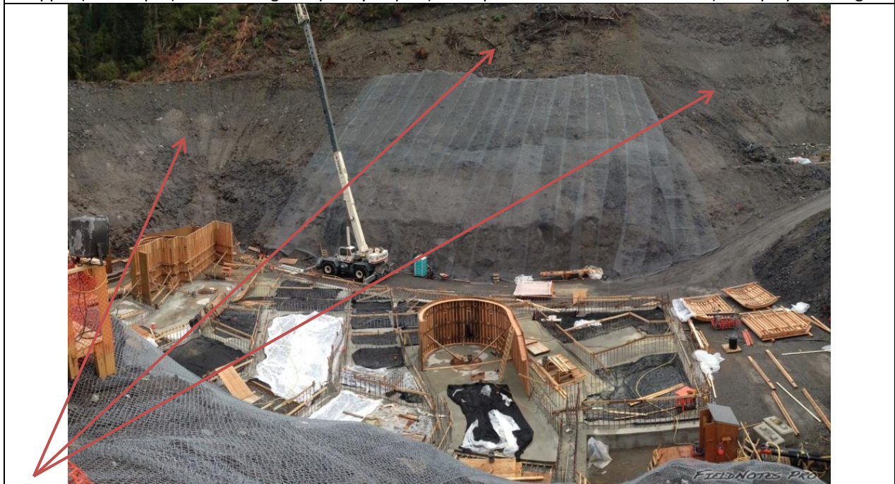
Photo 18. Slope stabilization measures required at the ULRHEF powerhouse cut slopes to protect against erosion. Recommendations include the application of hydro-seed with appropriate mulch product (BFM or FGM) for the upper (final slopes) and covering temporary slopes (below powerhouse backfill elevation) with poly-sheeting.
