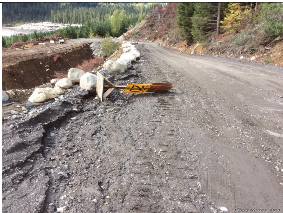
Photo 16. Road grading and ditch installation along the length of the camp access road/pebble main (~1.25km) is required to direct and convey road surface runoff to prevent further erosion. Check dams installation is recommended in steeper sections to prevent ditch line erosion and permit sediments to drop out of suspension.
