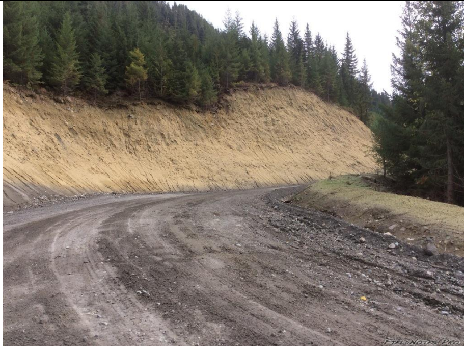
Photo 11. Ditch improvement, road grading to direct surface runoff to the ditch line, and slope erosion protection (to prevent further rill erosion) is recommended at the start of the Truckwash Creek FSR realignment (~42.75 km).
