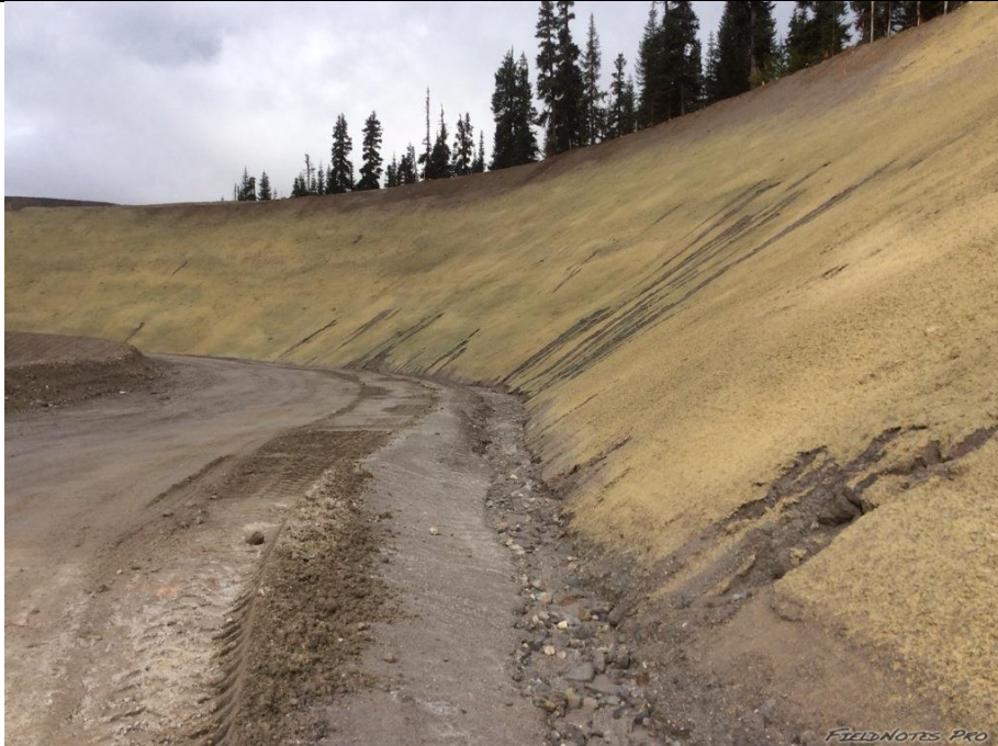
Photo 3. Rilling and gully erosion forming on the north side/upstream portal excavation cut slopes. The installation of velocity dissipation slope breaks to slow surface runoff or the application of a hydro-mulch better suited to the slopes (BFM or FGM) is recommended. Ditches should be cleaned and check dams installed/maintained as required. Erosion of the ditch line is not currently achieving intended ESC goals.
