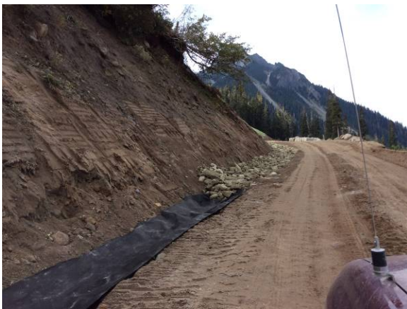
Photo 7 – Ditch lining and armoring of Lillooet River FSR on south side of ULRHEF intake (October 3, 2014).
