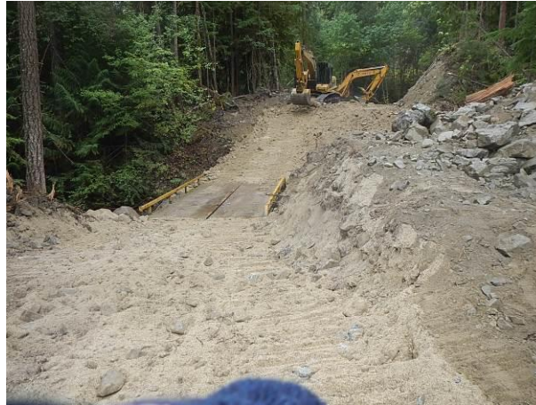
Photo 17 – Work on the right bank approach for the permanent Black Creek Bridge (September 23, 2014).
