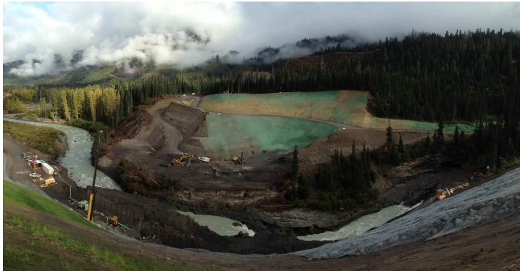
Photo 1 – Overview of the north side of the ULRHEF intake. Hydro-seed was applied to slopes as a temporary ESC measure (September 27, 2014).
