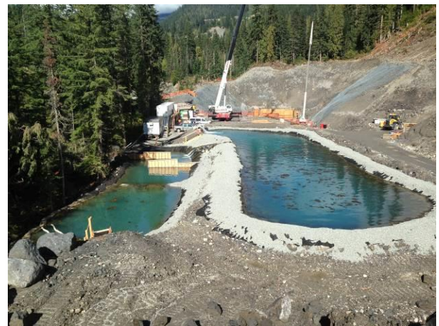
Photo 2 – Settling ponds at ULRHEF powerhouse, dewatering from excavation remains isolated from concrete works (September 27, 2104).
