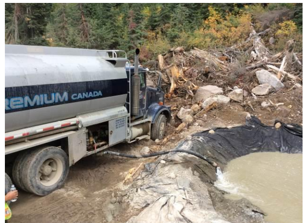
Photo 3 – Hauling water to infiltration pit during grouting works within the Obermeyer weir footprint (September 22, 2014).
