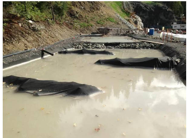
Photo 14 – BDRHEF powerhouse settling pond, no discharge observed; however pond #1 is now full of sediment and requires maintenance. (September 27, 2014).
