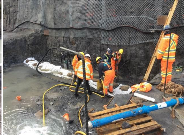
Photo 5 – Water management during grout work in isolated section of Obermeyer weir excavation. The blue pipe is the CO 2 injection/static mixer used for pH adjustment. Water as tested and confirmed to be below pH 9 prior to reaching the pump (September 24, 2104).
