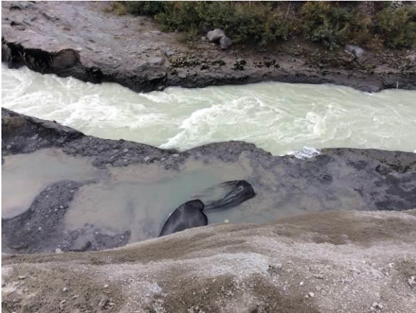
Photo 4 – ULRHEF intake diversion channel, dewatering bag for seepage control during grouting works (September 23, 2014).
