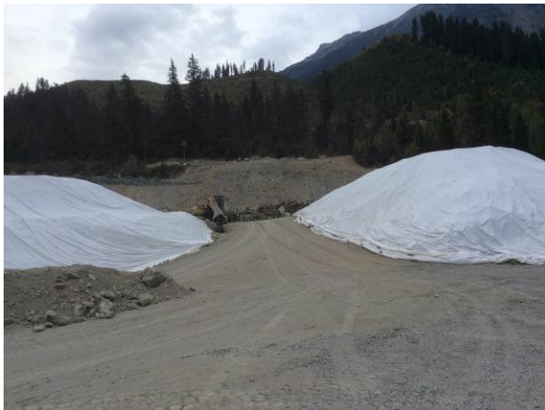
Photo 7 – Temporary PAG stockpiles located near the ULRHEF downstream tunnel portal were covered with impermeable plastic tarps (September 15, 2014).
