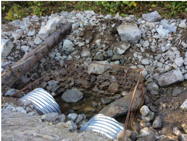
Photo 15 – South Lillooet FSR – Beaver exclusion fencing installed at the inlet of the doubled 1000mm culverts (September 15, 2014).
