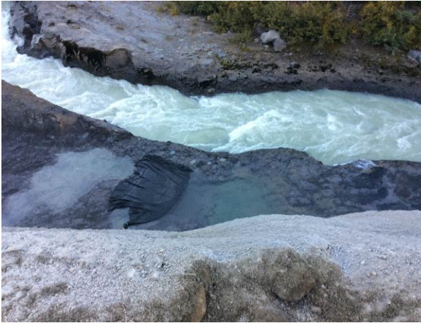
Photo 3 – ULRHEF intake diversion channel, dewatering bag for seepage control during grouting works (September 20, 2014).
