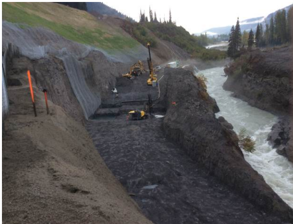
Photo 1 – Continued excavation of ULRHEF intake diversion channel, within the Obermeyer weir footprint (September 20, 2014).
