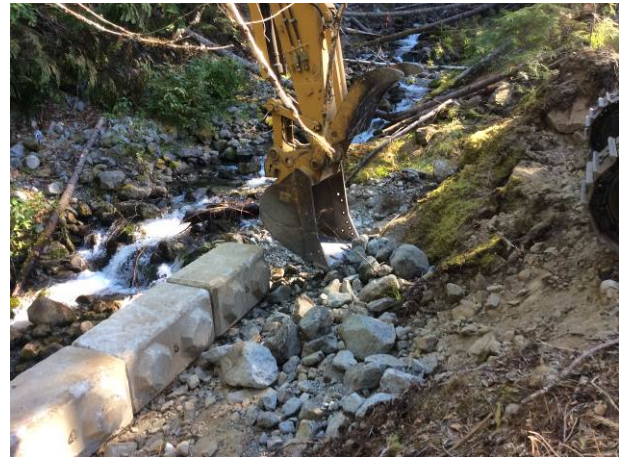
Photo 16 – Excavator installing temporary bridge footing at Blacks Creek Temporary Bridge. No instream works were required (September 15, 2014).
