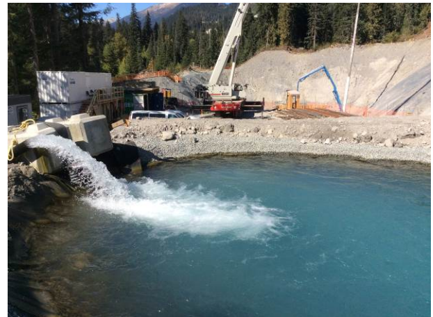
Photo 10 – Settling ponds at ULRHEF powerhouse, dewatering from excavation remains isolated from concrete works (September 16, 2104).
