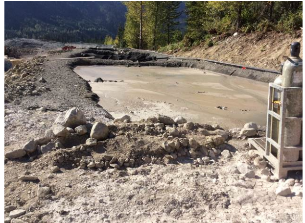
Photo 14 – BDRHEF powerhouse settling pond, no discharge observed; however pond #1 is now full of sediment and requires maintenance. (September 16, 2014).
