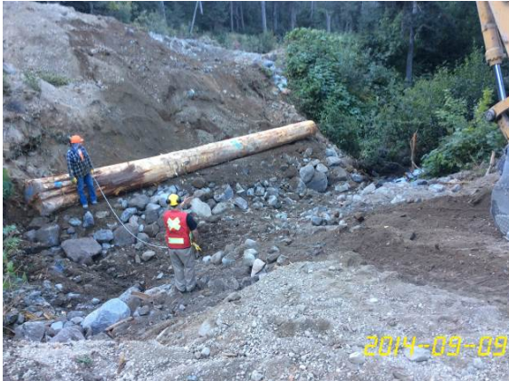
Photo 17 – Lillooet River FSR KM 47 log box culvert repair, placement of abutment timbers in isolated works area (September 9, 2014).
