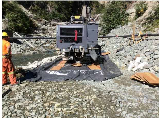
Photo 8 – Geotechnical drilling adjacent to Truckwash Creek, sandbag berm and secondary containment (September 12, 2014).
