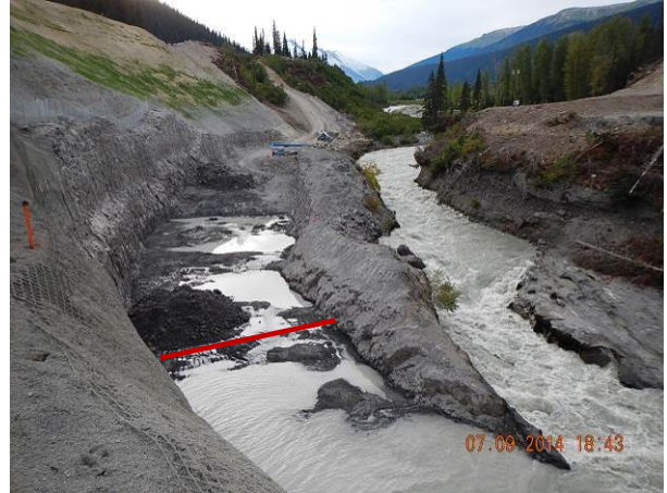
Photo 2 – ULRHEF intake diversion channel, backwatering due to elevated river flows (September 7, 2014)
