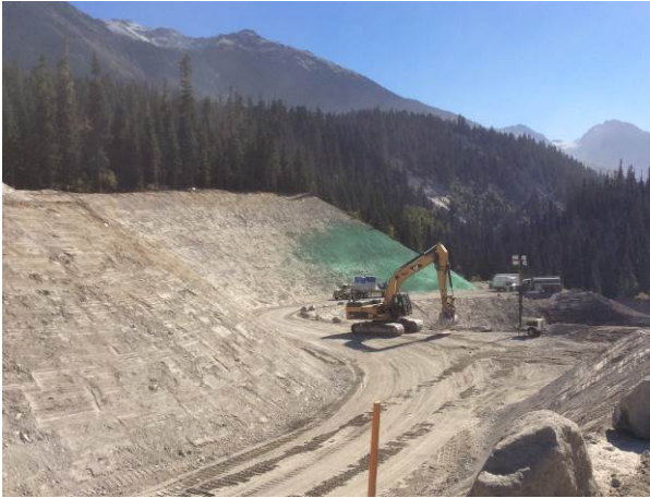
Photo 5 – Hydroseeding on final slopes adjacent to ULRHEF intake north side open cut bulk excavation (September 12, 2014)
