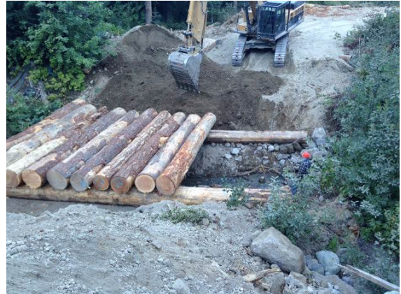
Photo 18 – Lillooet River FSR KM 47 log box culvert repair, partial rewatering occurred once ISW were completed (September 10, 2014).
