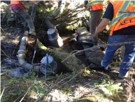
Photo 19 – Lillooet River FSR KM 39.7 box culvert repair, sand bag diversion installation of two 6" pumps fitted with fish screens (September 11, 2014).
