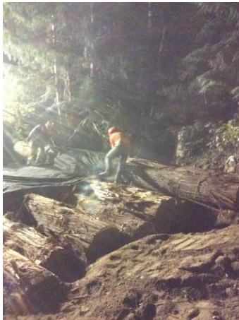
Photo 21 – Lillooet River FSR KM 39.7 box culvert repair, abutment logs and stringer placement within isolated works area (September 12, 2014).
