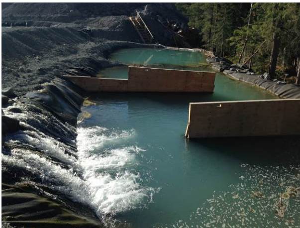
Photo 13 – Settling ponds at ULRHEF powerhouse, dewatering from excavation remains isolated from concrete works (September 10, 2014).
