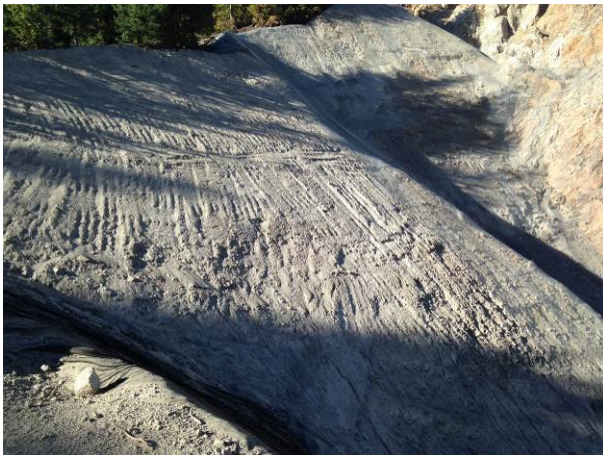
Photo 9 – ULRHEF downstream tunnel portal cut slopes requiring hydroseeding or other erosion mitigation (September 9, 2014).
