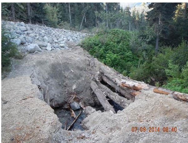
Photo 15 – KM 47 log box culvert prior to repair works (September 7, 2014)
