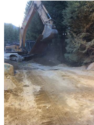
Photo 20 – Lillooet River FSR KM 39.7 box culvert repair, removal temporary road plates (September 11, 2014).
