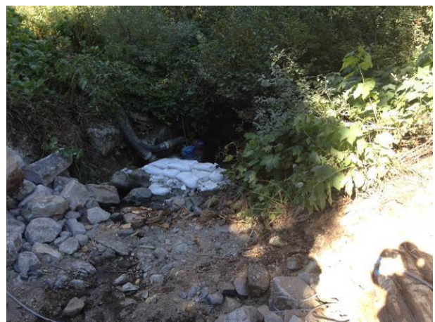
Photo 16 – Sandbag diversion berm and two 6” pumps fitted with fish screens at KM 47 log box culvert repair (September 9, 2014).
