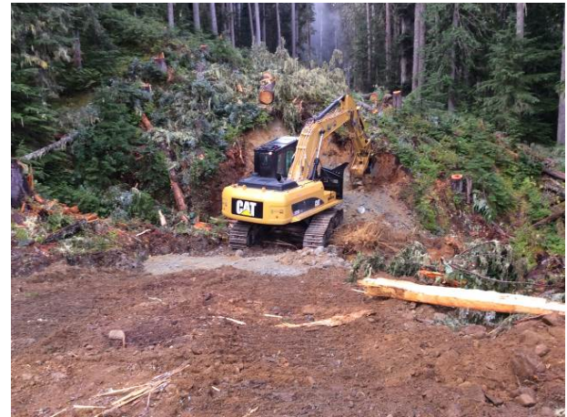
Photo 15 – Construction commenced along access road 371.1, excavator grubbing area for box culvert near dry creek bed (September 2, 2014)
