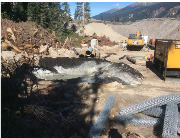
Photo 5 – Concrete wash out pit in spoil area on south side of Lillooet River at ULRHEF intake (September 4, 2014).
