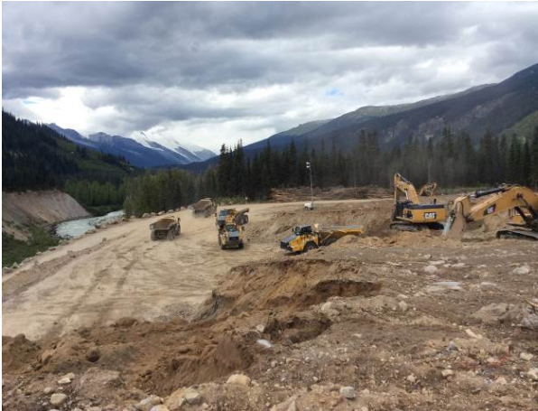
Photo 3 – Commencement of bulk excavation at the ULRHEF intake open cut on the north side of the Lillooet River (August 31, 2014)
