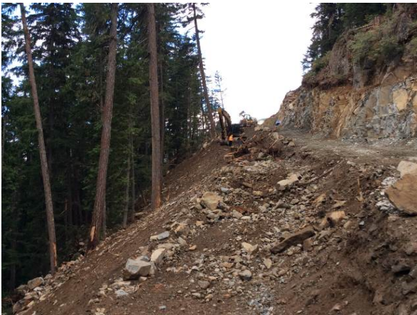
Photo 8 – BDRHEF Intake access road construction including slope contouring and LWD/boulder removal from toe of slope (August 31, 2014)
