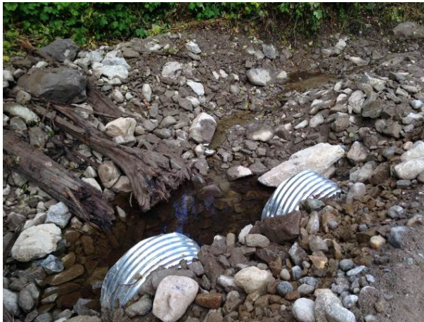
Photo 14 – Two 1000 mm culverts installed at 6km on the Lillooet South FSR (September 3, 2014).
