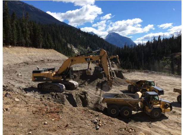
Photo 4 – Continued bulk excavation at the ULRHEF intake open cut on the north side of the Lillooet River (September 3, 2014).
