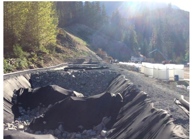
Photo 11 – Settling ponds and pH treatment at BDRHEF tunnel portal (September 6, 2014)
