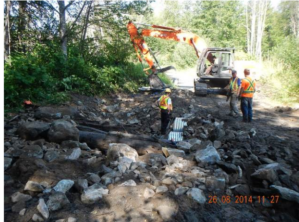
Photo 13 – Installation of two 1000 mm culverts at 6 km on the Lillooet South FSR (August 26 th , 2014).
