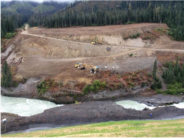
Photo 9 – Stripping and grubbing on north side of Lillooet River at intake (August 30 th , 2014)
