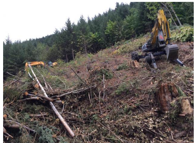
Photo 11 – Segment 5 machine works (excavator and spider hoe) at structure locations (August 30 th , 2014).
