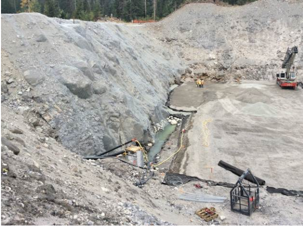
Photo 5 – Powerhouse excavation showing French drain in construction, back fill and compaction (August 25 th , 2014)
