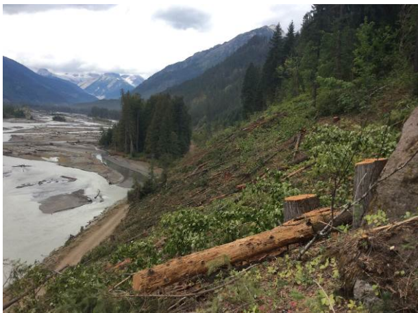
Photo 10 – Segment 5 steep slope falling (August 29 th , 2014).
