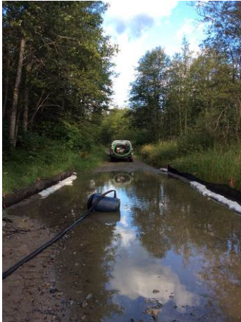
Photo 12 – Continued dewatering of salvaged and isolated wetted areas to vegetation prior to road ballasting (August 28 th , 2014).
