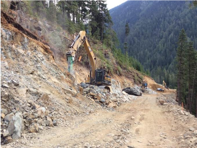
Photo 1. Completing slope stabilization along the new Boulder Intake access road following prescription outlined in the work plan. (August 21, 2014).
