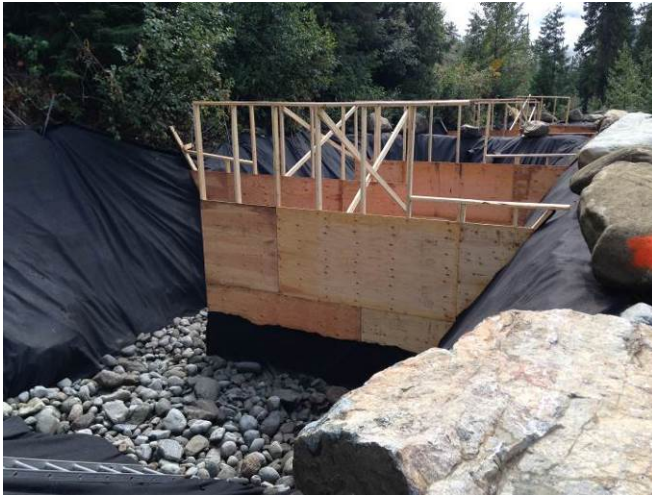
Photo 3. Constructed sediment ponds to be used for treatment of seepage water emanating from the ULRHEF downstream tunnel portal. (August 15, 2014).
