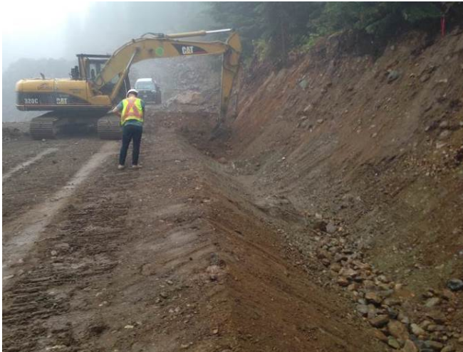
Photo 1. Ditching and slope stabilization along the new Boulder Intake access road following prescription outlined in the work plan. (August 15, 2014).
