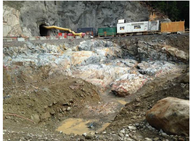
Photo 2. Dewatering of seepage from within the powerhouse excavation was pumped to the sediment ponds. Water has not yet reached the second treatment pond (August 15, 2014).
