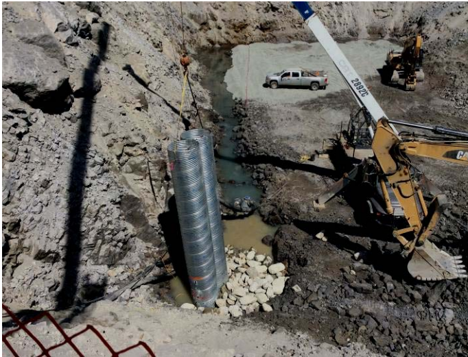
Photo 3. Installing sumps within the ULR powerhouse excavation. Water is running as clean as the Lillooet River but will continue to be directed to the treatment ponds (August 7, 2014).
