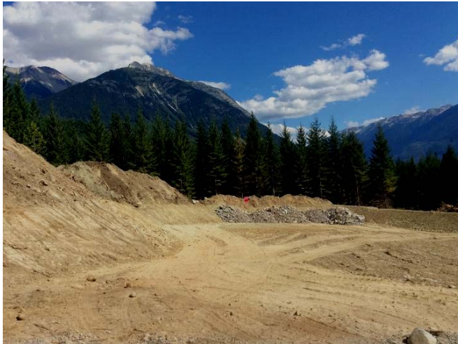
Photo 1. Preparing BDR-4 as a temporary storage area for PAG generated from the Boulder Intake access road construction. This area will be used once works resume following the removal of the Stop Work Order (August 6, 2014).
