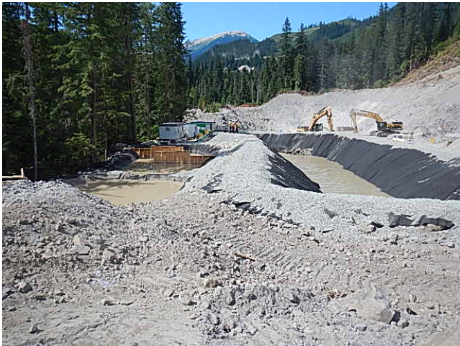
Photo 3. New large sediment pond constructed for the dewatering of the ULRHEF powerhouse excavation (August 1, 2014).
