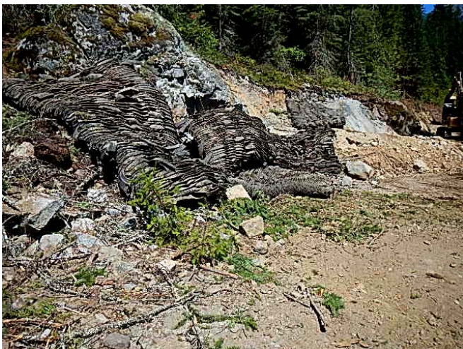
Photo 5. Blast mats placed prior to blasting at the Ryan River bridge approach. (August 1, 2014).
