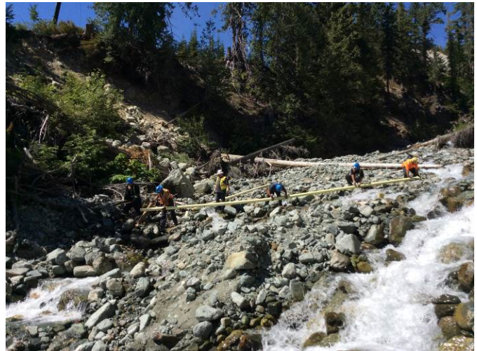
Photo 4. Installation of the gravity feed water diversion system within Truckwash Creek. Water will be used for construction activities at the ULR downstream portal. (July 27, 2014).
