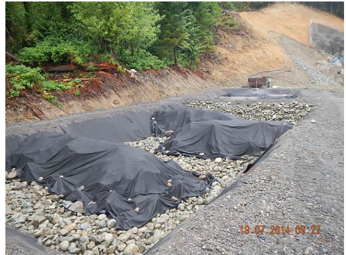
Photo 2. Dewatering of seepage from the tunneling activities was performed this week but the water has not yet reached the second pond treatment pond (July 19, 2014).
