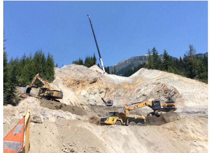
Photo 4. Excavation and mesh installation at the ULRHEF downstream tunnel portal location (July 14, 2014).
