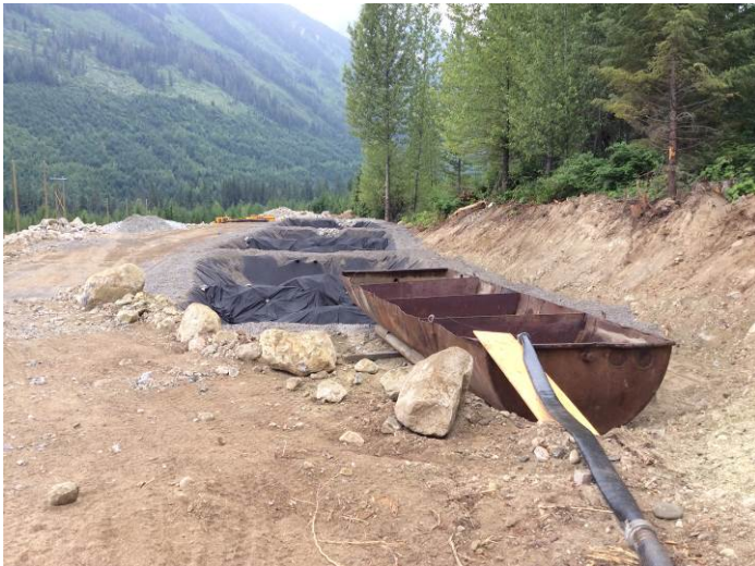
Photo 1. Series of three settling ponds at the BDRHEF downstream tunnel portal work area. (July 4, 2014).
