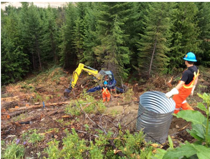
Photo 5. Pole foundation installation in Segment 2 with an excavator capable of working on steep slopes (July 5, 2014).
