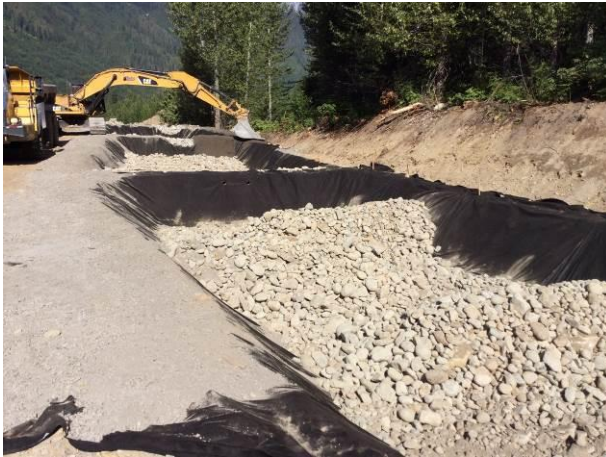
Photo 1. Installing the series of settling ponds at the BDRHEF downstream tunnel portal work area. (June 26, 2014).
