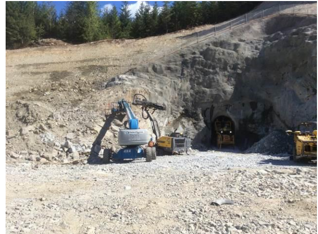
Photo 2. Rock bolt stabilization and tunneling works at the tunnel portal entrance. (June 26, 2014).
