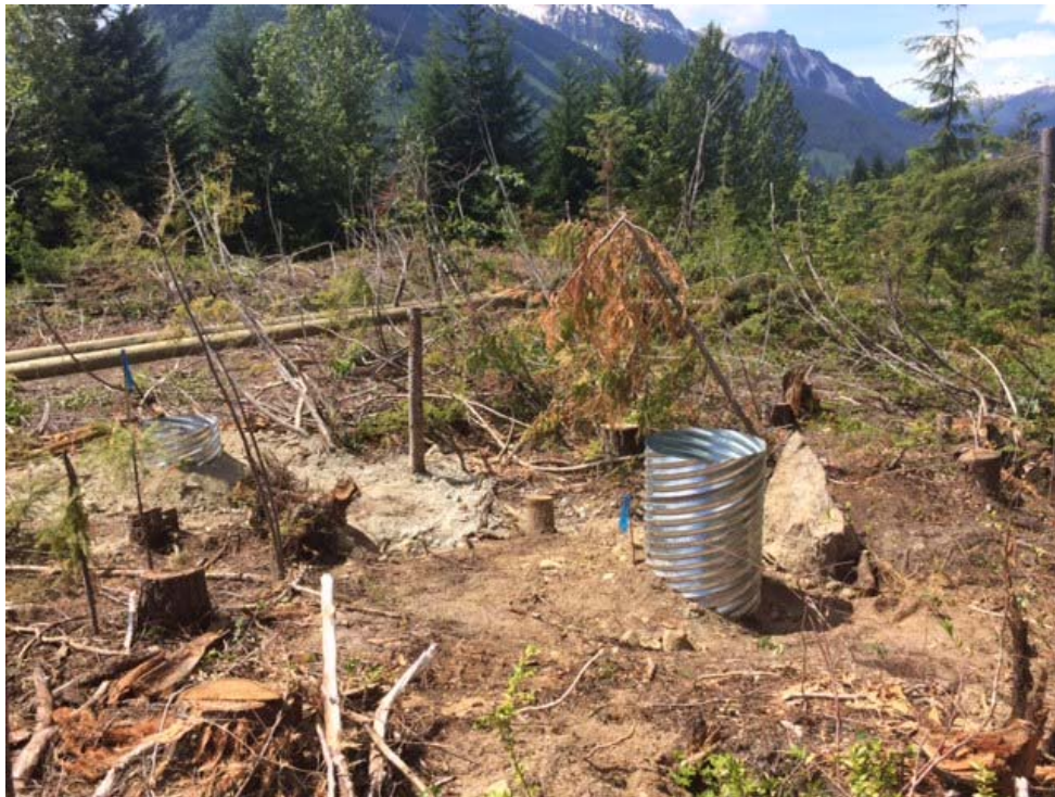
Photo 2. Taken on June 25, 2014, from outside of the RVMA, showing culvert liners installed along the edge and within the RVMA.
