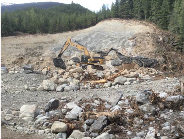
Photo 1. Placing blast mats at the BDRHEF downstream portal location prior to blasting (June 12, 2014).
