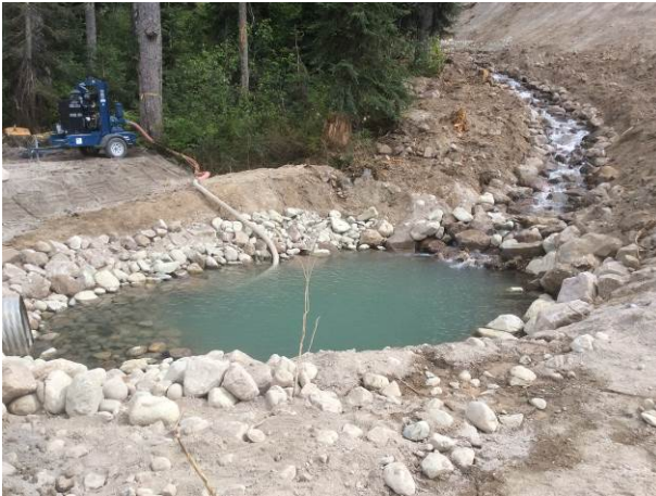
Photo 4. Conditions following the diversion of the spring fed creek through the newly constructed diversion channel (June 12, 2014).
