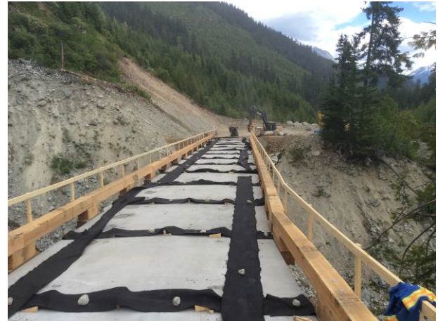
Photo 5. The Truckwash Creek bridge during curing of the grout installed on June 12 th (June 14, 2014).
