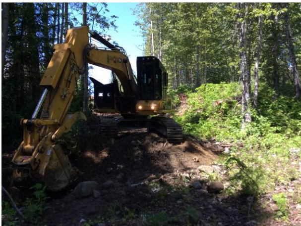
Photo 6. Culvert installation work proceeding in the dry; Pebble D.1 Branch road (June 5, 2014).
