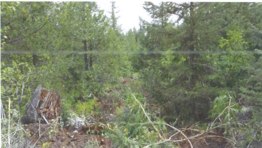
Photo 3: Access track where CRT-ebc excavator walked in to the site to remove rock truck.
