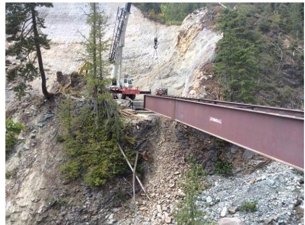
Photo 5. Launch of the Truckwash Creek bridge girders from the east abutment. (June 6, 2014).
