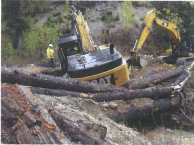
Photo 1: The CRT-ebc 45 tons excavator, moments after the box culvert collapsed.
