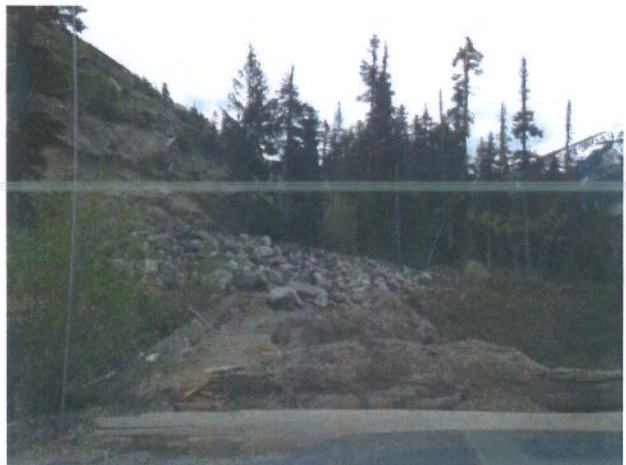
Photo 4: The slope above the creek was stabilized with boulders to avoid sediment from entering the watercourse.
