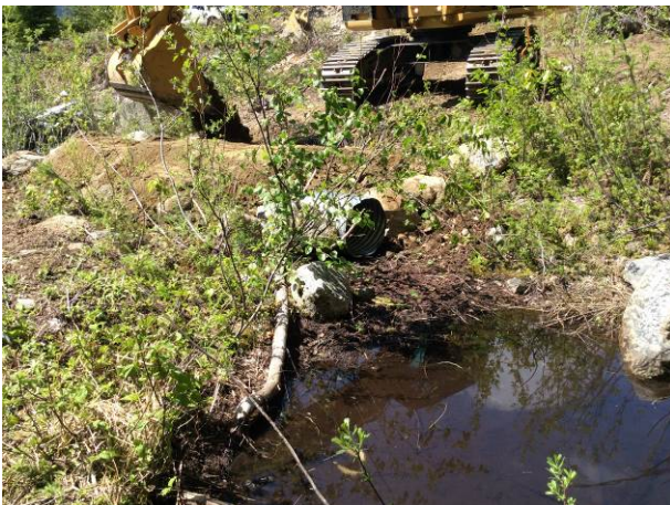
Photo 6. Dewatering of the work area during the culvert installation; Pebble D.1 Branch road (May 20, 2014).
