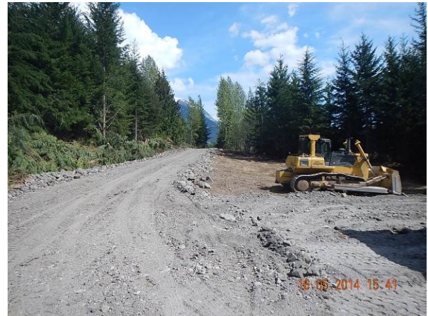
Photo 2. Upgraded section of the access road (01/2.1) to the Explosive magazine area. (May 16, 2014).
