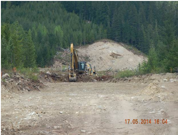
Photo 1. Rough grading of the BDRHEF powerhouse access road works. The stripped and grubbed portal location can be seen in the background (May 17, 2014).
