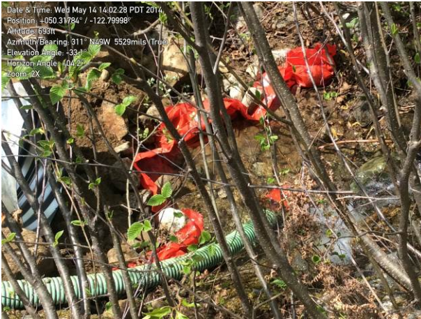
Photo 5. Intake hose installed to divert stream 35b around the active work area during the culvert installation (May 14, 2014).
