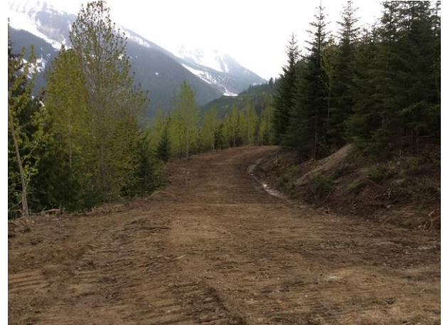
Photo 2. Upgraded section of BDRHEF intake access road following ditch installation and tree removal. (May 8, 2014).
