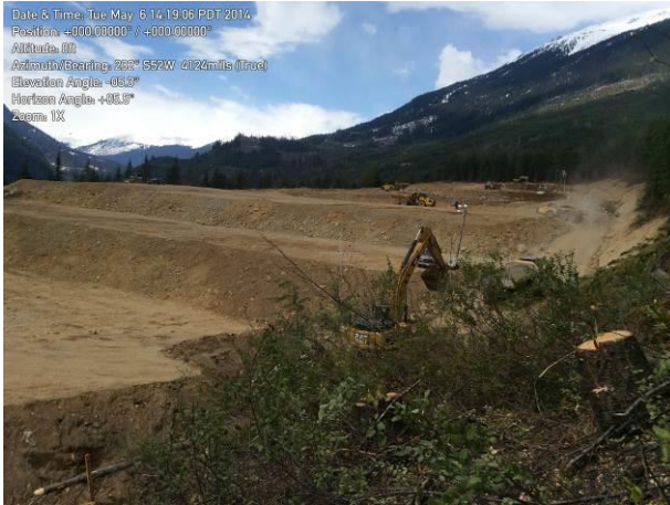
Photo 1. Nearing completion of site grading and sub-grade preparation at the Construction Camp work area. (May 6, 2014).
