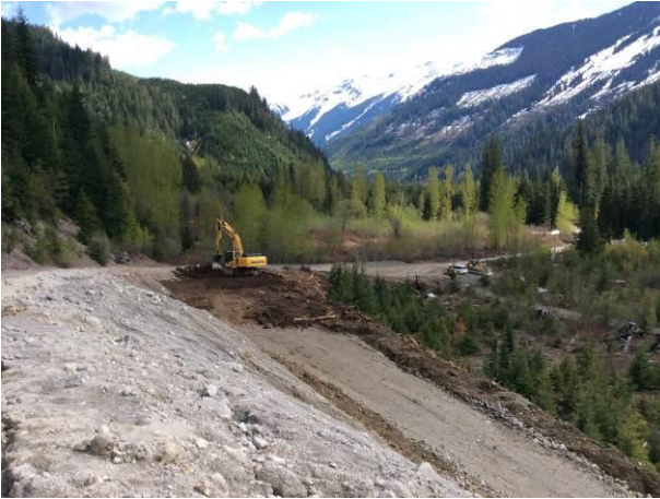
Photo 3. Placing stripping and grubbing material from the ULRHEF powerhouse area work area at the base of the approved spoil area. (May 10, 2014).
