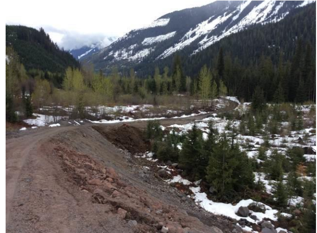
Photo 4. Stockpiling of organic material from the ULRHEF powerhouse at the base fill slope at the east heading of the Truckwash Creek realignment. (May 3, 2014).
