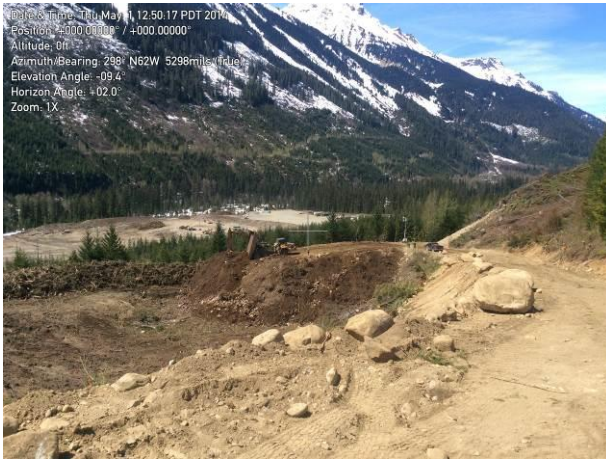
Photo 1. Stockpiling stripping and grubbing material from the Construction Camp work area. Note the separation of woody debris and organic soils (May 1, 2014).
