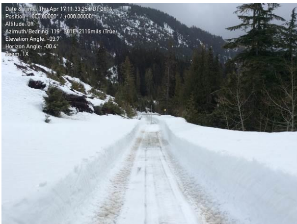
Photo 1. Overview of the snow removal works at 45km of the Lillooet River FSR. (April 17, 2013).
