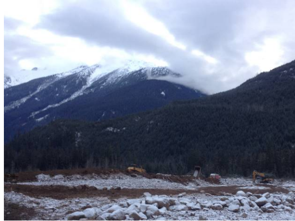
Photo 4. Construction of the visual/auditory berm at the future construction camp location. (Dec 11, 2013).
