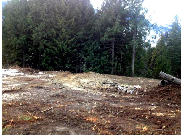
Photo 2. Additional cross ditching installed across the road grade at the east heading of the Lillooet River FSR realignment (outside of the Truckwash Creek Mountain Goat Migration Corridor). (Nov.26, 2013)
