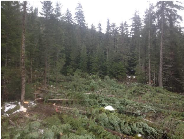
Photo 5. Results of clearing within the Boulder Creek Powerhouse footprint. Looking towards the future tail race location (Nov.28, 2013).
