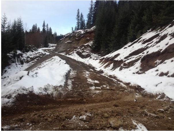
Photo 1. Two cross ditches installed across the road grade at the east heading of the Lillooet River FSR realignment (outside of the Truckwash Creek Mountain Goat Migration Corridor). (Nov.26, 2013).
