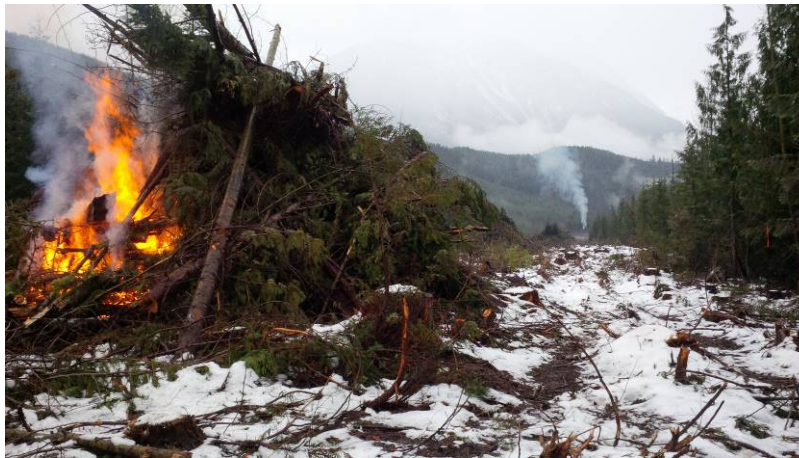
Photo 5. Burning debris piles between Poles 10 – 12 (Nov 15, 2013).
