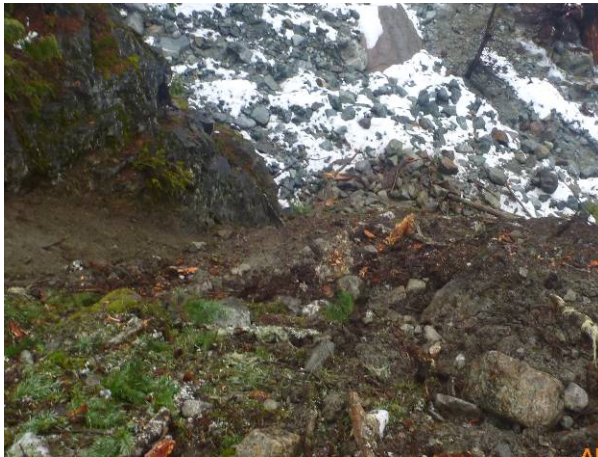
Photo 1. Boulder debris that fell during excavation of the right bank bridge abutment. The IEM was onsite during the excavation work adjacent to Truckwash creek on Nov 14, 2013.
