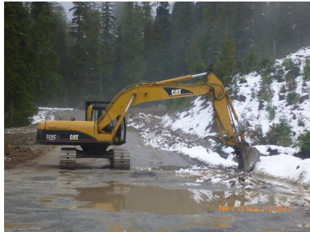
Photo 2. Ditching on the at the west heading of the Truckwash Creek FSR realignment as part of winterization measures (Nov.12, 2013).
