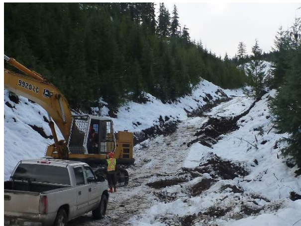
Photo 2. Ditching and cross ditching installed along completed section of road alignment on the east heading of Truckwash Creek. Work was completed as part of winterization of the site. (Nov 8, 2013).
