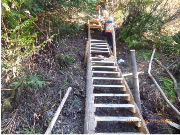
Photo 3. Construction of stairs required for a steep section of the trail. (Oct. 25, 2013).
