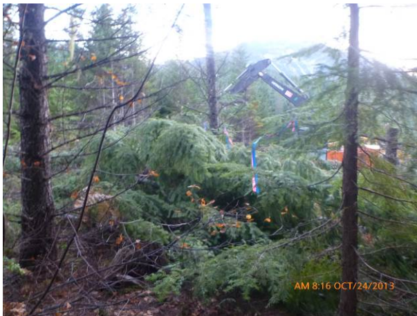
Photo 5. Clean-up activities within 15m of Boulder Creek. Notice the pink and blue flagging that delineates the 15m RVMA area. Equipment did not pass this line during clean-up works (Oct. 24, 2013).
