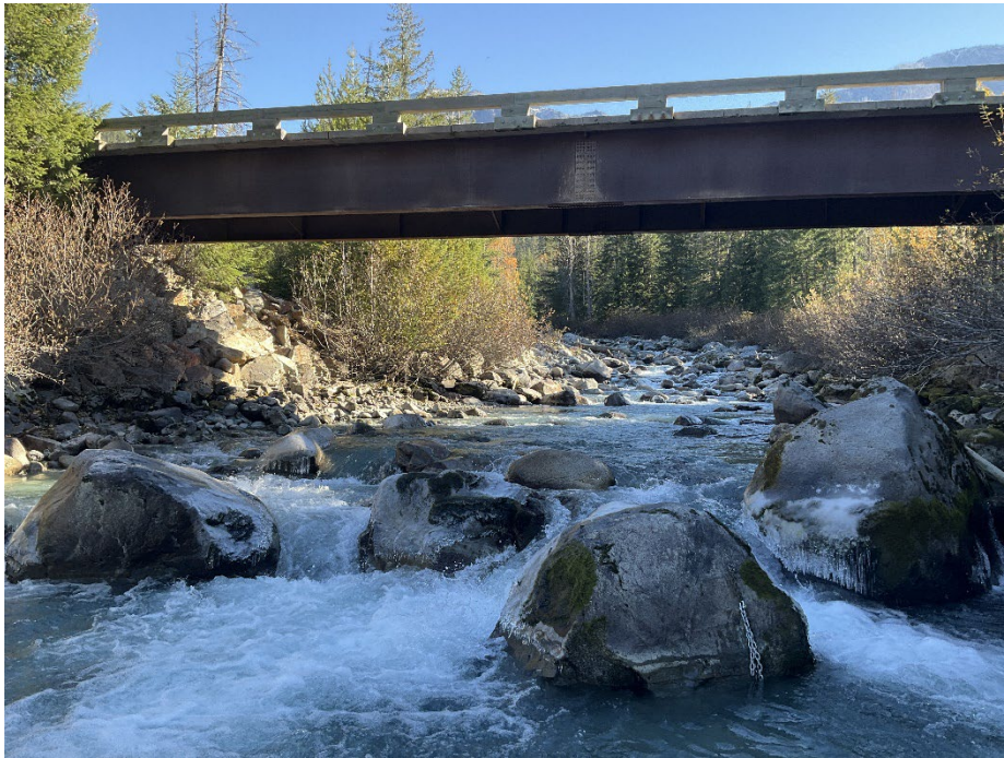
Figure 30. Looking upstream at Tidbit 1 at BDR-DSWQ on October 28, 2023.
