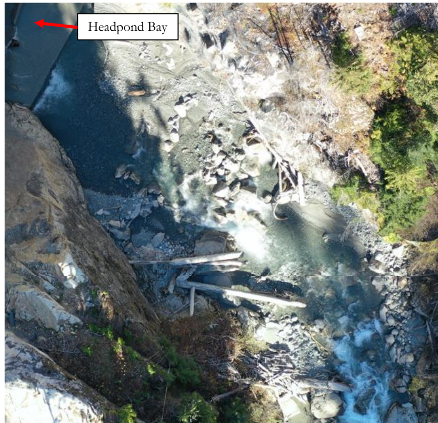
Figure 21. Evidence of large wood and spawning gravel being transported below the Boulder Creek headpond bay on October 28, 2023.
